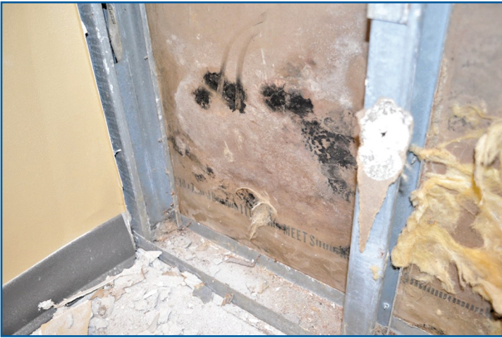
Figure 15 – Mold growth on the interior side of exterior sheathing.
