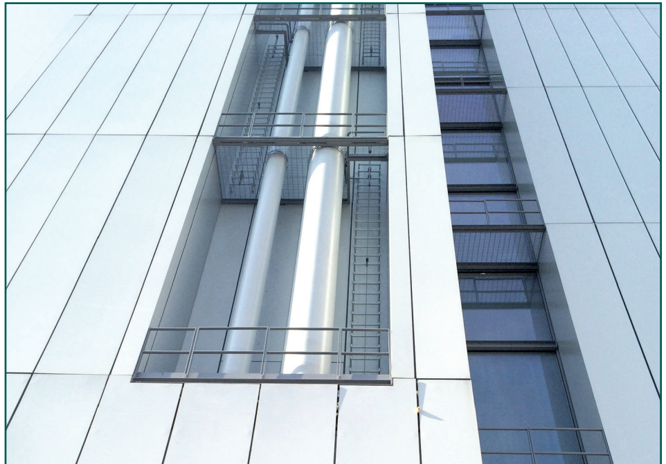
Figure 3 – Example of a ladder safety system.
