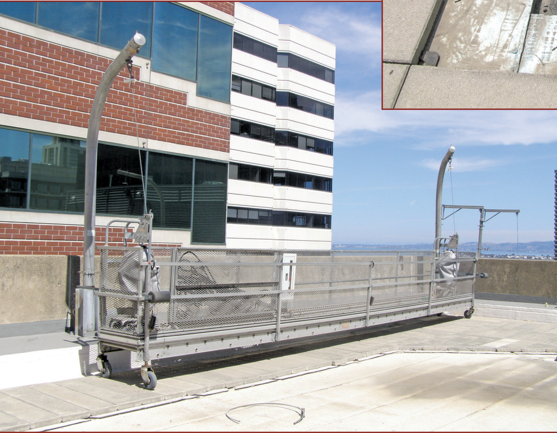
Figure 2 – Typical davit-supported work platform.
