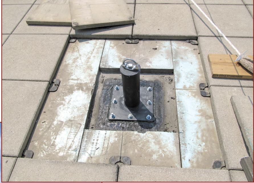
Figure 3 – Anchorage on a roof.
