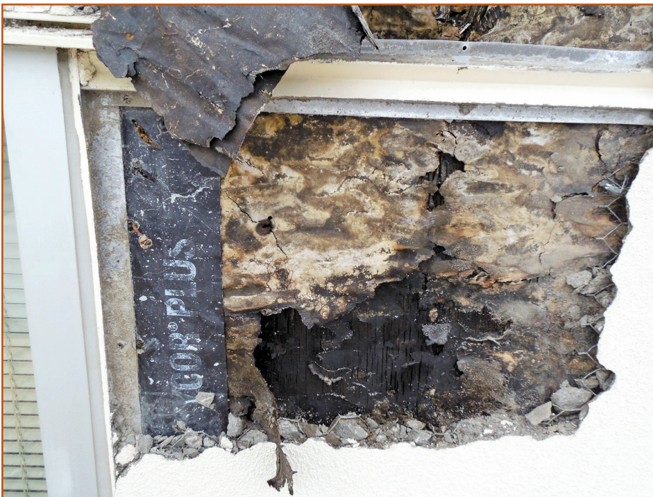
Photo 5 – Water infiltration through the exposed fasteners exacerbates resulting damage at the stud framing and sheathing.
