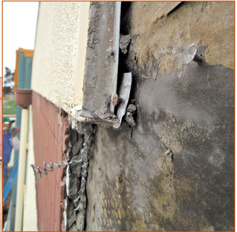
Photo 4 – The bugle-headed self-drilling tapping screws sit proud of the vertical reveal and the horizontal casing bead.
