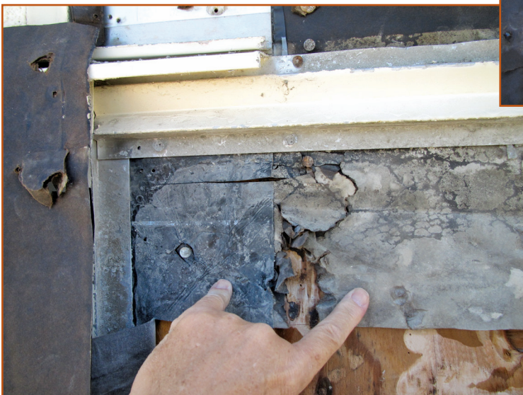
Photo 14 – The two layers of ripped and deteriorated building paper correspond to the corroded tapping screw above.
