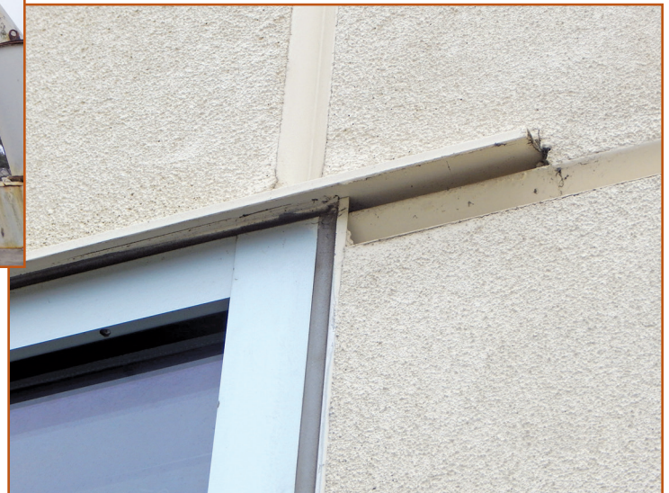
Photo 9 – Nozzle spray testing (see Photo 8 ) at this corner of the window frame rapidly caused interior leakage at the sill.
