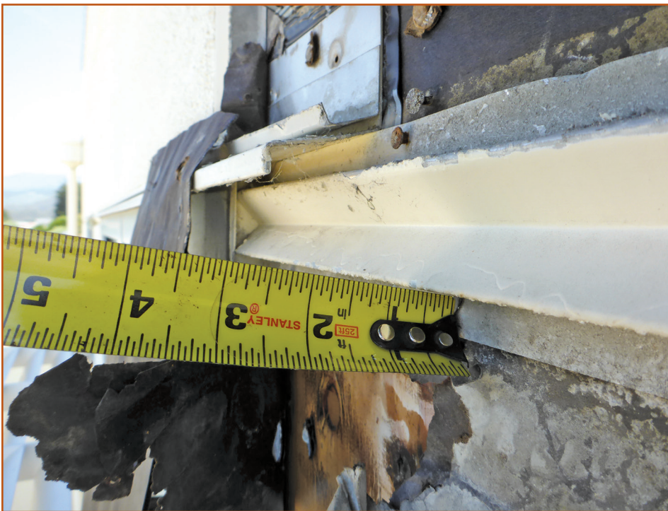
Photo 16 – The linchpin of this entire deleterious water-intrusion process was the improperly installed self-drilling tapping screw projecting from the horizontal reveal.
