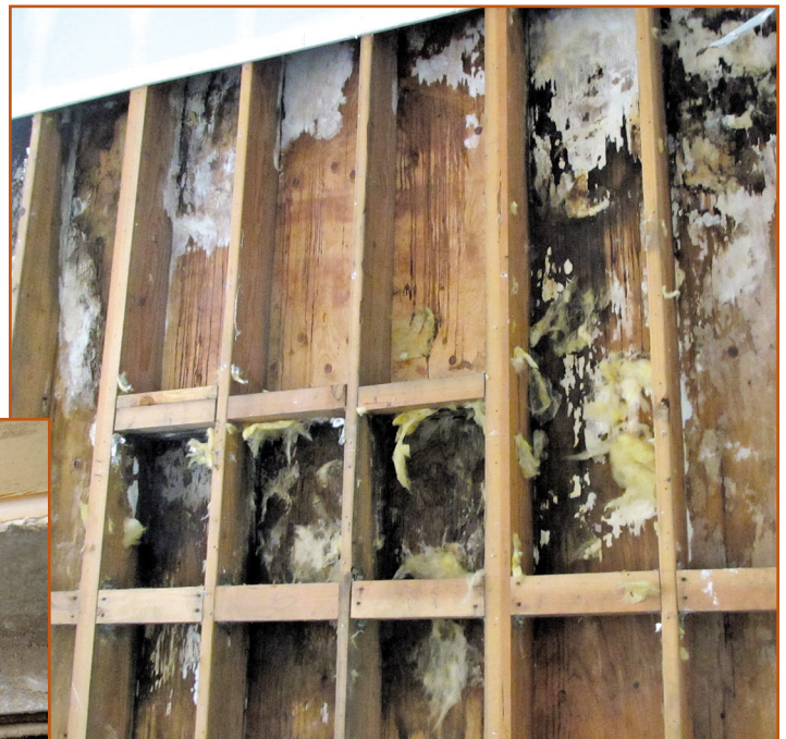
Photo 1 – Building envelope failures at this school building have resulted in extensive deterioration and fungal growth within weather-exposed wall assemblies.
