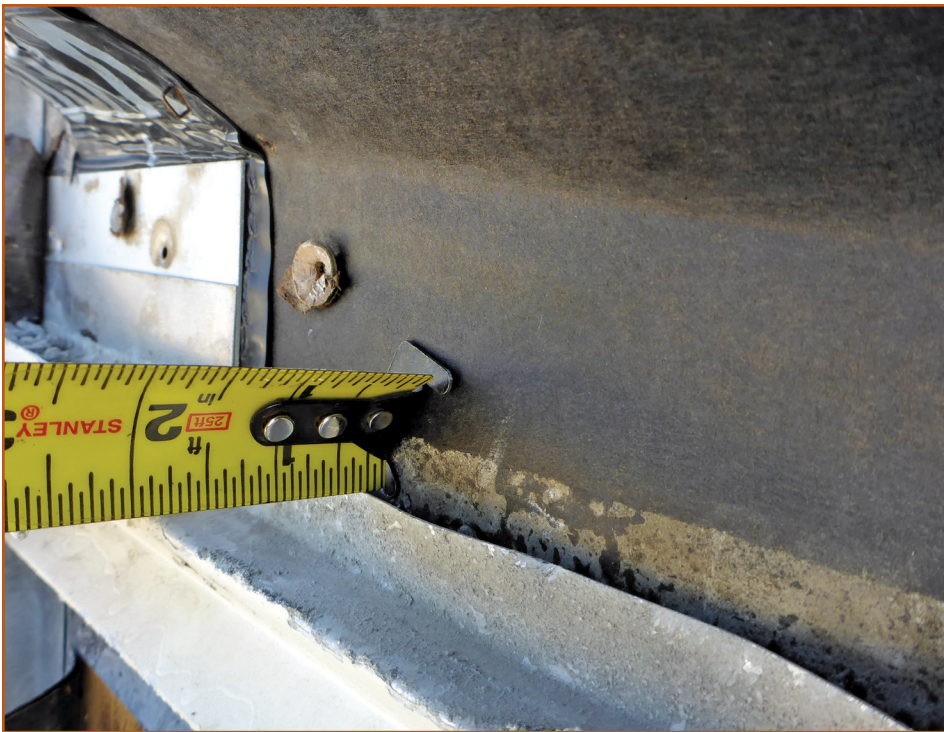
Photo 17 – Rainwater drainage off the head flashing and J-mold accessory had immediate access behind this loosely set reveal.
