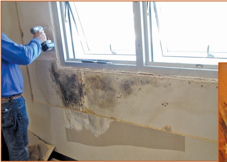
Photo 6 – Wet, degraded (and fungal-contaminated) gypsum wallboard layers were exposed below an upper window.
