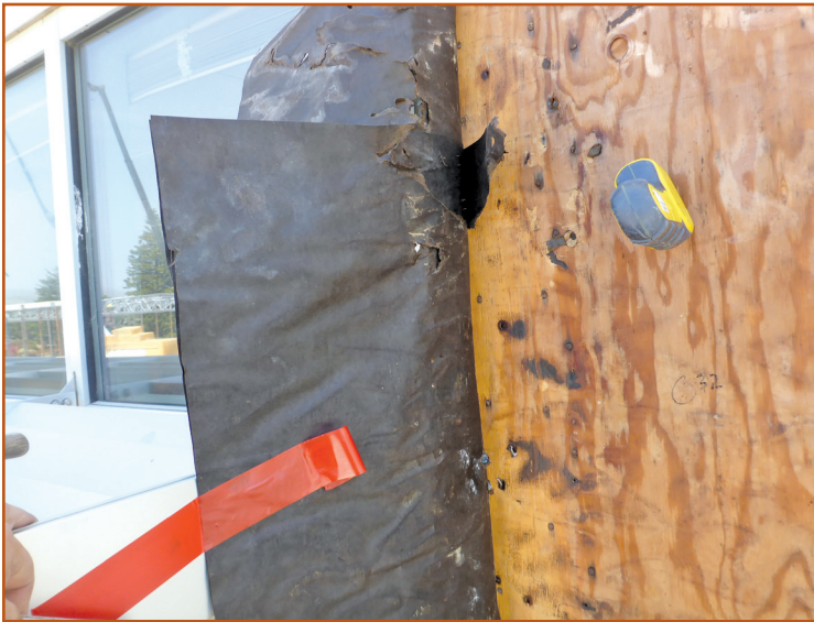
Photo 11 – We traced the water trail up the wall toward the window head (see Photo 12).
