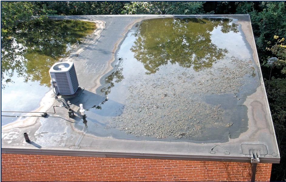
Figure 8 – This hollow-core deck has experienced creep during service life and now exhibits negative camber between the interior bearing walls. It can certainly occur in other deck types, but deformation of this nature can be perilous, especially during periods of rain on snow.
