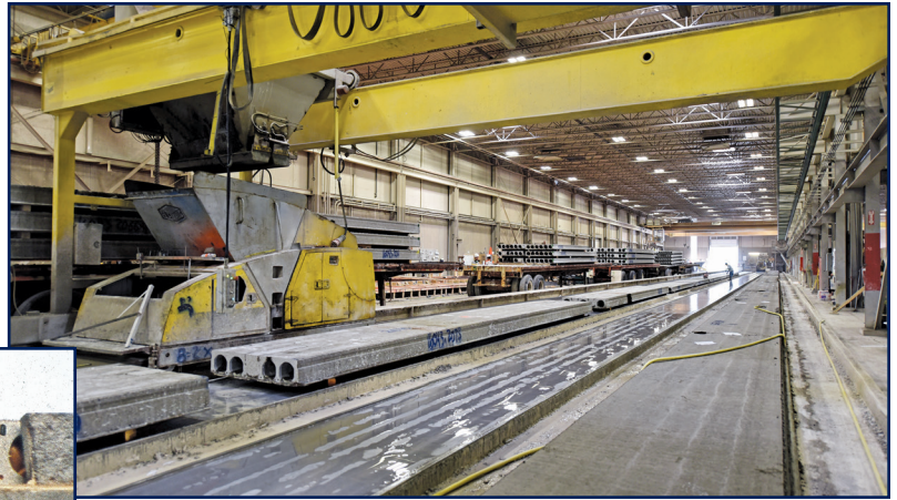
Figure 4 – The forms, also known as the “casting beds,” are prepared, after which the steel tendons are situated and stretched (stressed) prior to placement of the concrete. This image depicts a large indoor production facility (courtesy of Kerkstra Precast, Grandville, MI).
