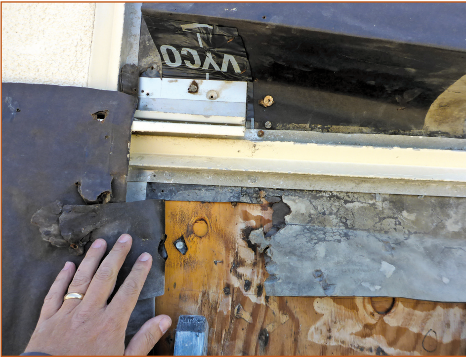
Photo 15 – The trail of water damage leads directly to the head flashing and J-mold accessory above the horizontal reveal.
