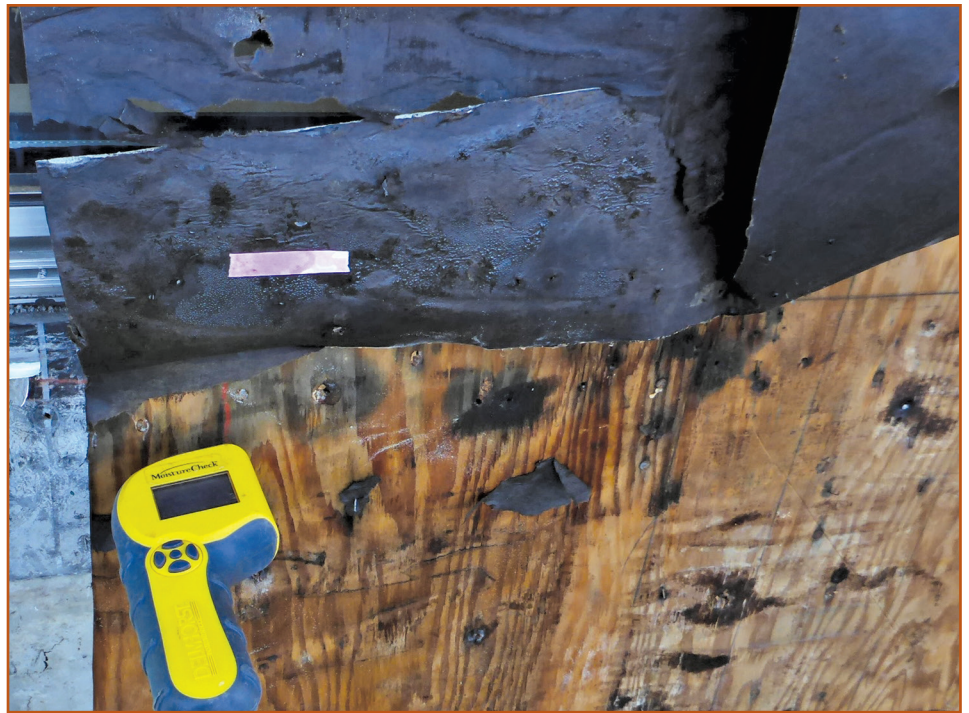
Photo 10 – Water-finding test paper turns red when in contact with free water.
