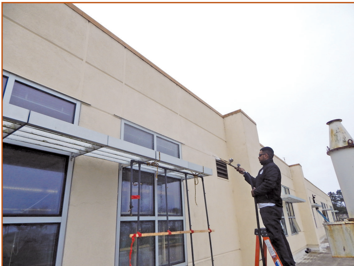
Photo 8 – AAMA nozzle testing at the upper right corner (see Photo 9 ) of this window produced interior leakage at the sill.
