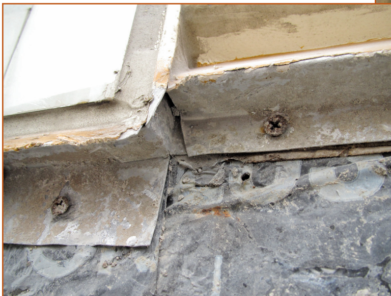
Photo 2 – Bugle-head “self-drilling tapping screws” were used to secure the stucco accessories and trim to the underlying plywood sheathing and wood framing.
