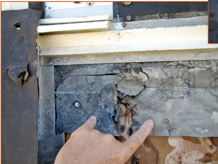
Photo 14 – The two layers of ripped and deteriorated building paper correspond to the corroded tapping screw above.
