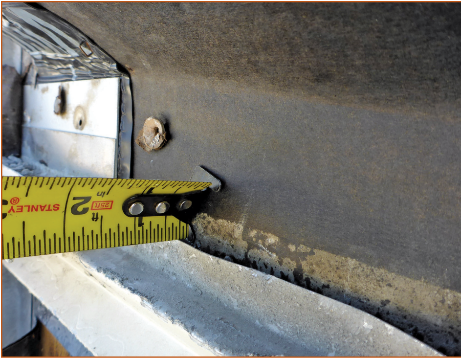
Photo 17 – Rainwater drainage off the head flashing and J-mold accessory had immediate access behind this loosely set reveal.
