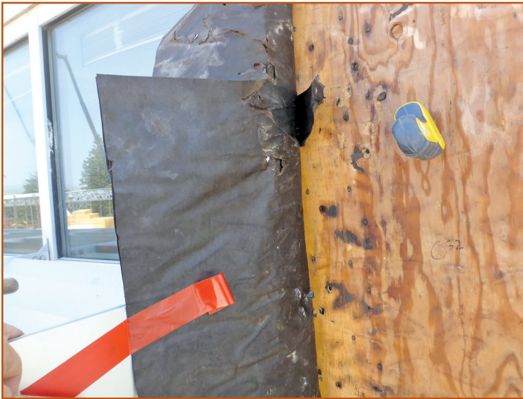
Photo 11 – We traced the water trail up the wall toward the window head (see Photo 12).
