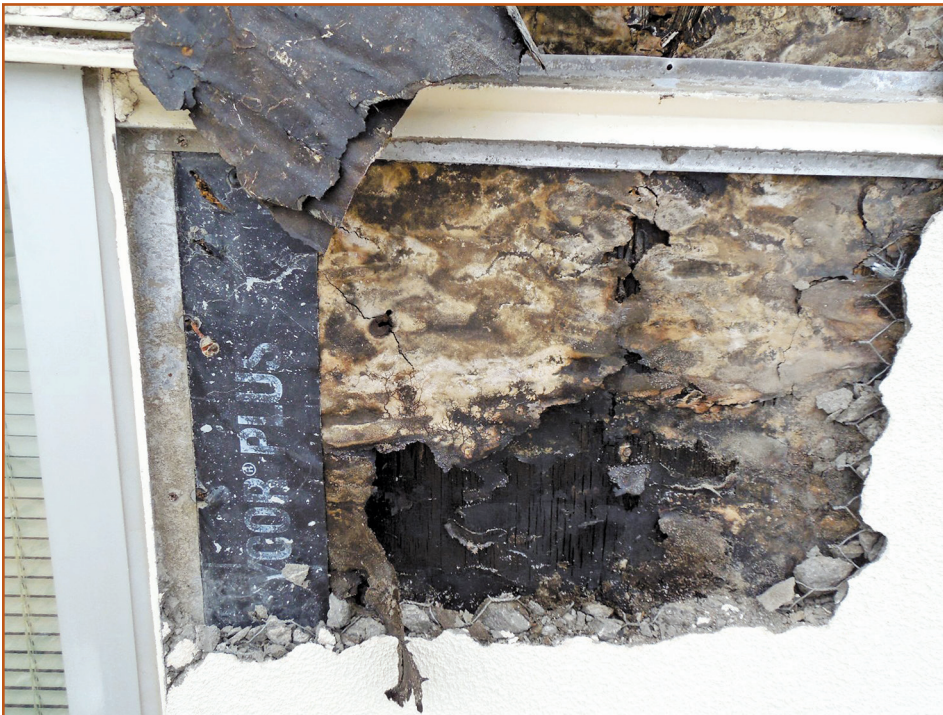
Photo 5 – Water infiltration through the exposed fasteners exacerbates resulting damage at the stud framing and sheathing.
