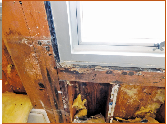
Photo 7 – Removal of the degraded wallboard revealed severely damaged framing and sheathing.
