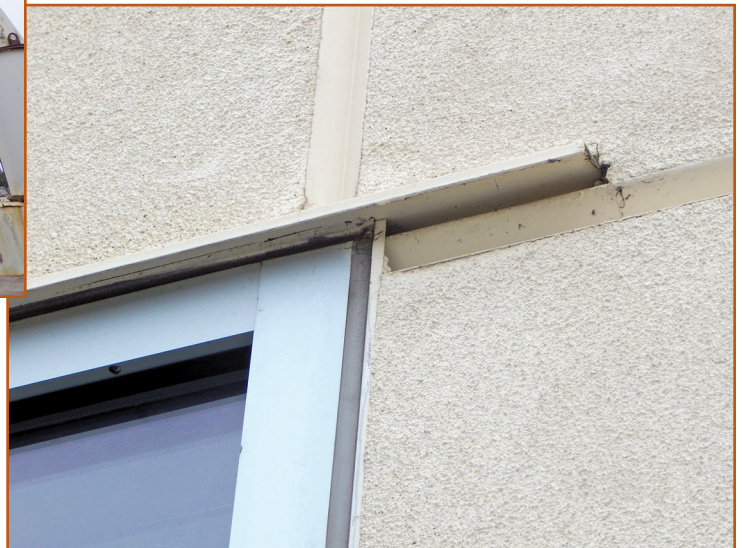
Photo 9 – Nozzle spray testing (see Photo 8 ) at this corner of the window frame rapidly caused interior leakage at the sill.
