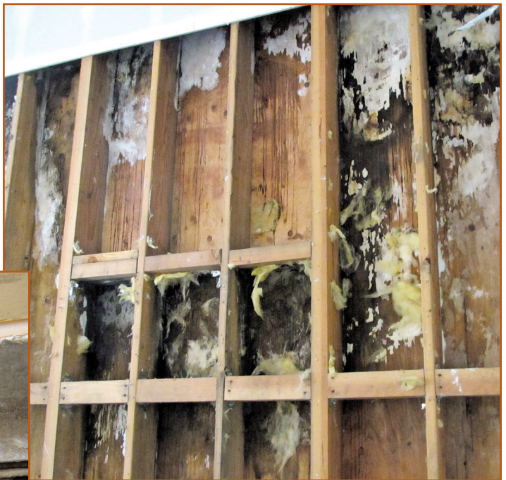
Photo 1 – Building envelope failures at this school building have resulted in extensive deterioration and fungal growth within weather-exposed wall assemblies.
