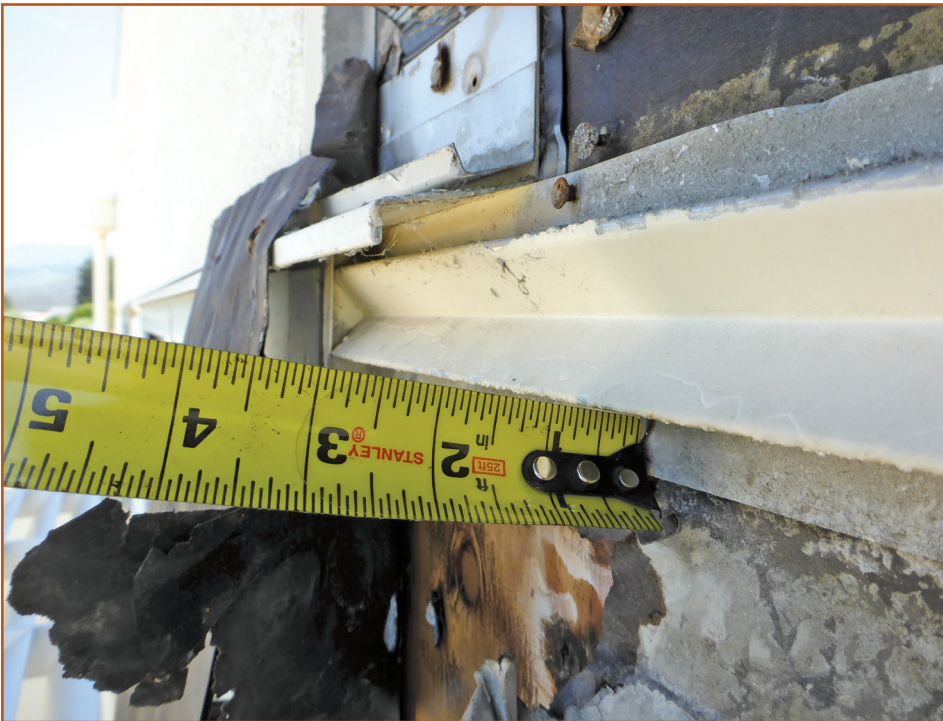
Photo 16 – The linchpin of this entire deleterious water-intrusion process was the improperly installed self-drilling tapping screw projecting from the horizontal reveal.
