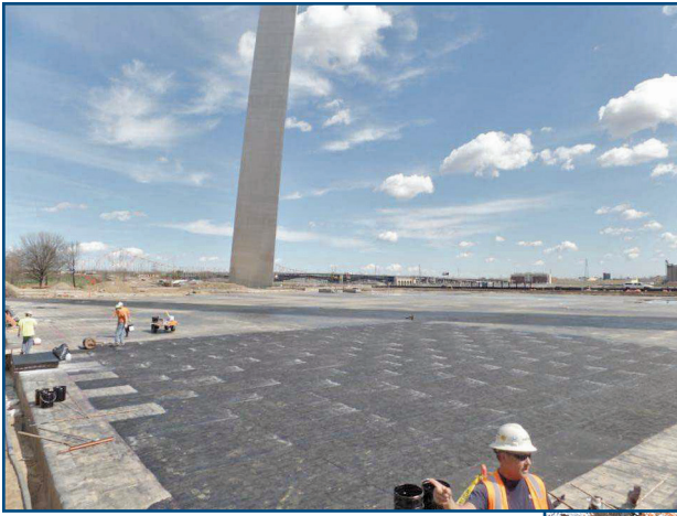
Figure 8 – A two-ply modified-bitumen sheet waterproofing membrane, an electronic leak detection system, and a permanent leak-detection grid system were installed on the museum roof beneath the historic Gateway Arch in St. Louis, MO.
