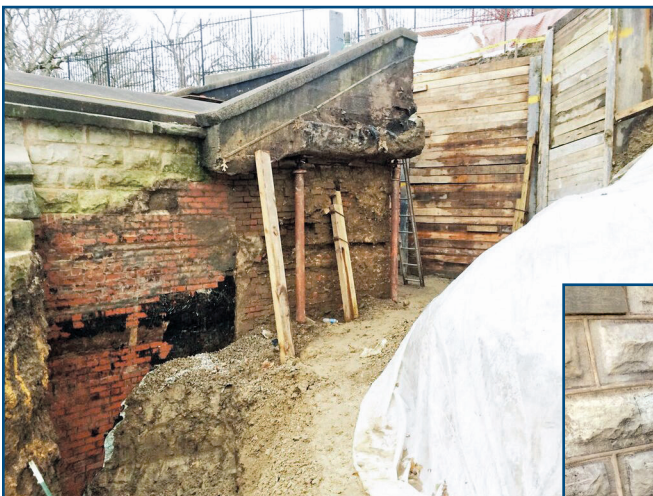
Figure 10 – The walls on the exterior of the vault were in very poor condition.
