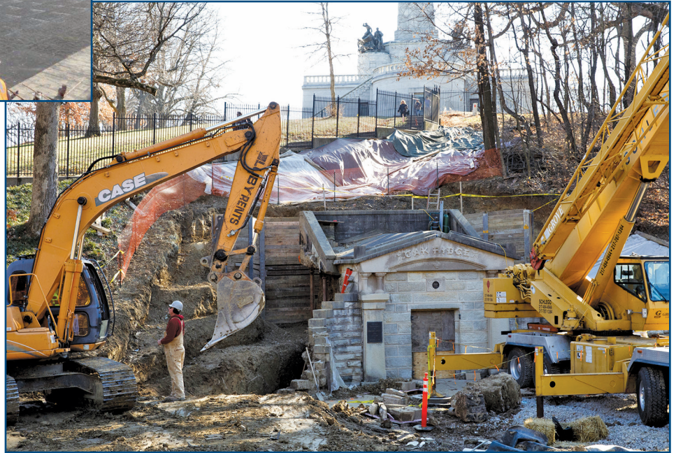
Figure 9 – The area around the Lincoln vault was excavated in preparation for waterproofing.
