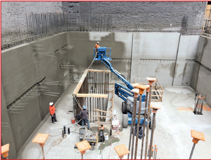
Figure 10 – The use of stay forms resulted in a change to negative-side waterproofing for this project.
