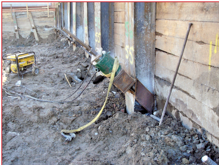
Figure 1 – Installation of tie-backs to support vertical piles occurs as the excavation proceeds downward.
