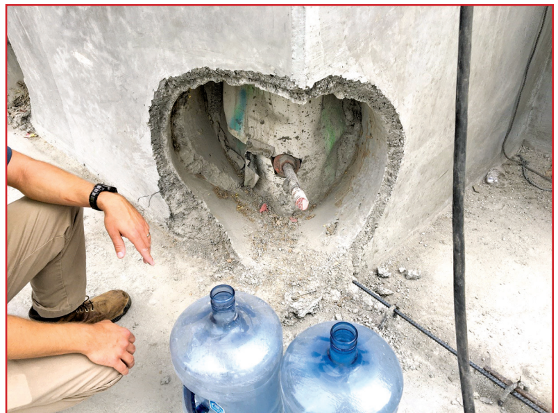
Figure 7 – This anchor rod will be cut back. Then the membrane and wall will be patched.
