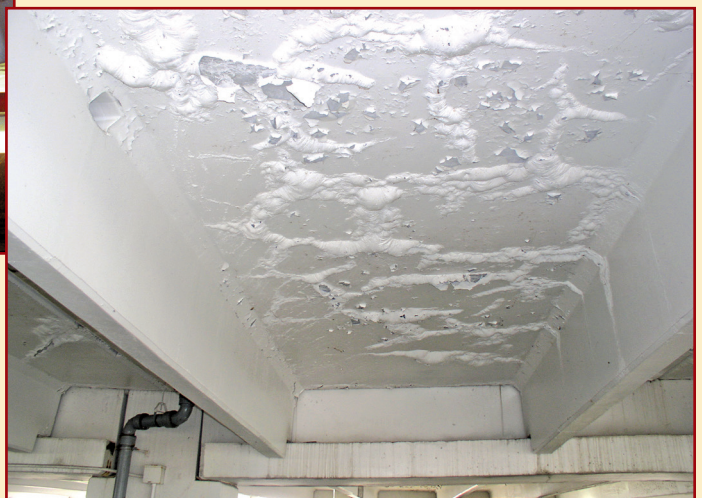
As water penetrated down through this elevated slab, it caused bubbling of the applied coating.
