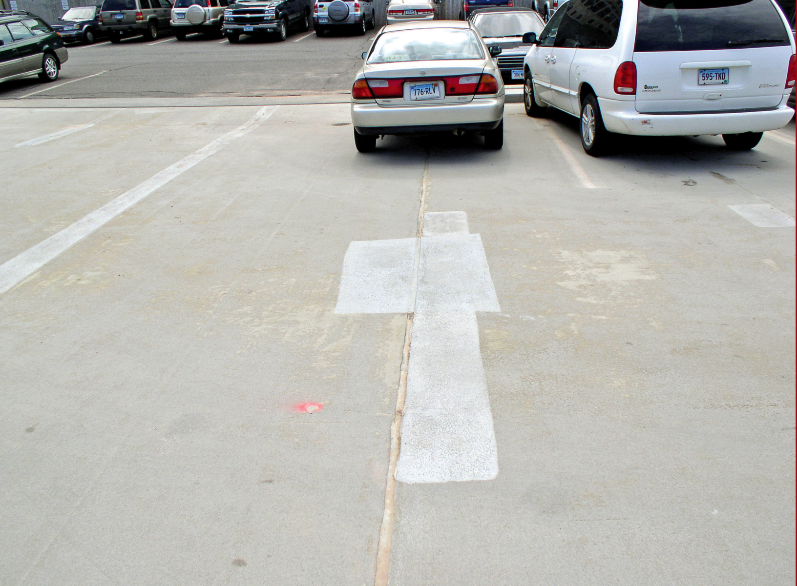
Figure 6 – Edges of pre-cast concrete units at sealant joints catch snowplow tips, quickly wearing away surface treatments. Here, coating patches were used as a temporary fix.
