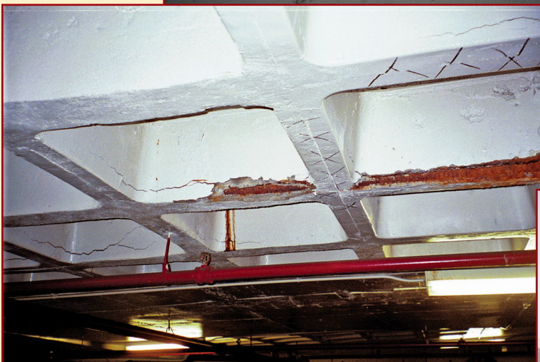
Surface spalling on an elevated deck may be a sign of trapped moisture.
