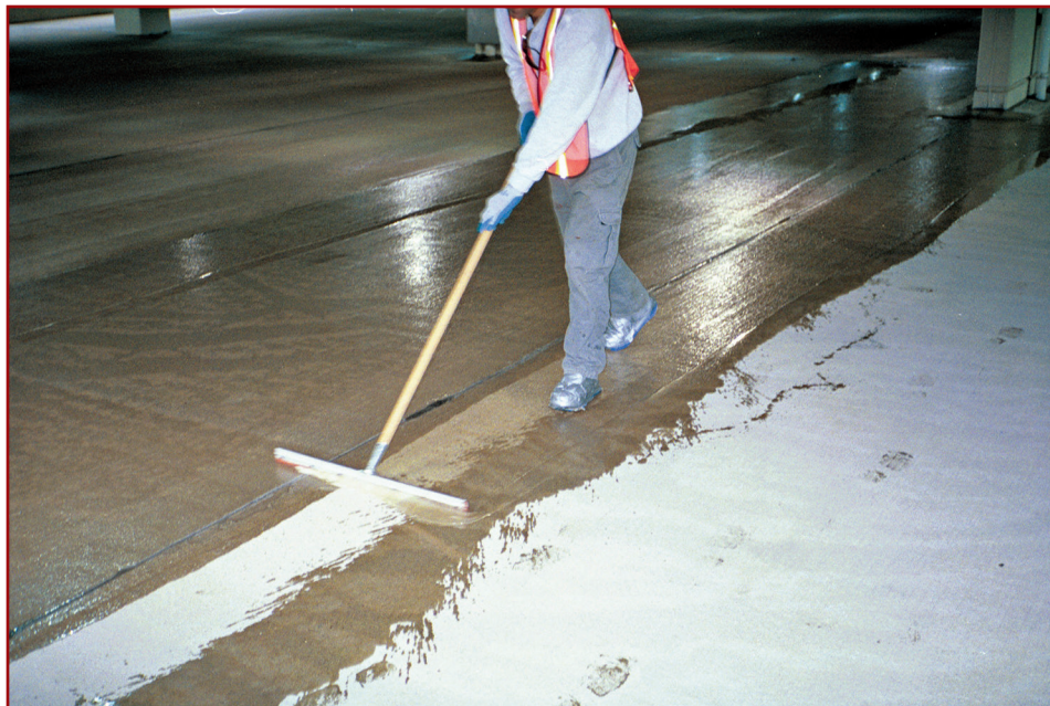
Figure 3 – Applying a low-cost sealer to a concrete deck can be a quick, effective, low-maintenance option.
