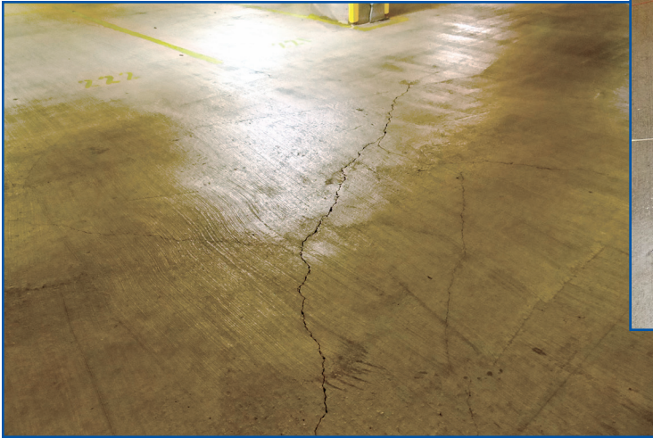
Figure 13 – Cracks in concrete.
