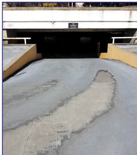
Figure 4 – Worn coating in high-wear turn area. These are areas that should be properly addressed during system design.
