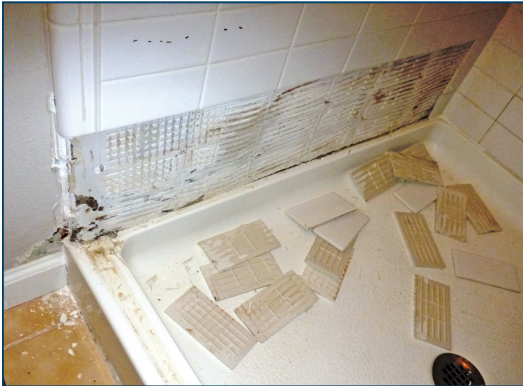
Figure 7 – Supplemental testing (at this purposefully selected shower) confirmed widespread water intrusion and extensive damage under loosely bonded ceramic tiles.
