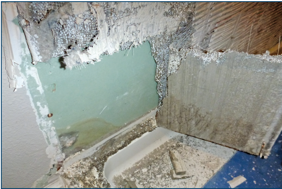
Figure 9 – Leakage and deterioration extended to the unprotected gypsum wallboard behind the CBU.
