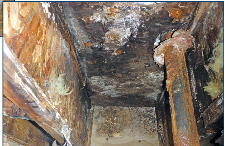
Figure 13 – The CBU butt joint leakage had destroyed the subfloor system and the underlying floor joists.
