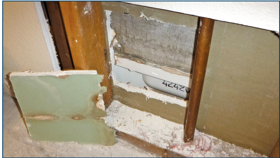
Figure 6 – Purposeful supplemental testing confirmed limited and localized water damage within this wall assembly.
