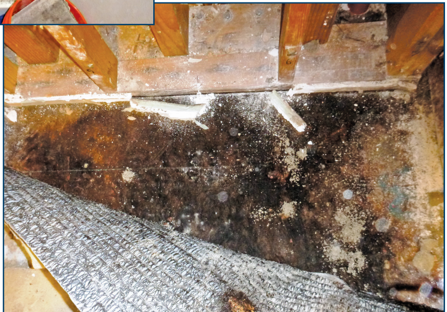
Figure 11 – The subfloor system below the fiberglass shower pan was also found to be severely damaged.
