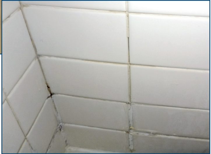
Figure 5 – At many shower walls at all three buildings, many of the grout joints were failing or missing.
