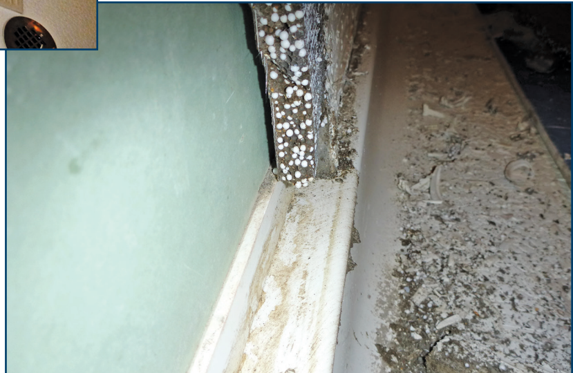
Figure 8 – As expected, the CBU panel was not properly lapped over the vertical flange.
