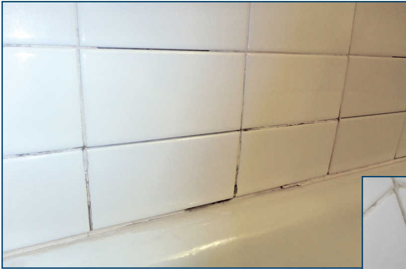
Figure 4 – Ceramic tiles at this tub-shower unit were loose. Multiple sections of the grout were deteriorated or missing.
