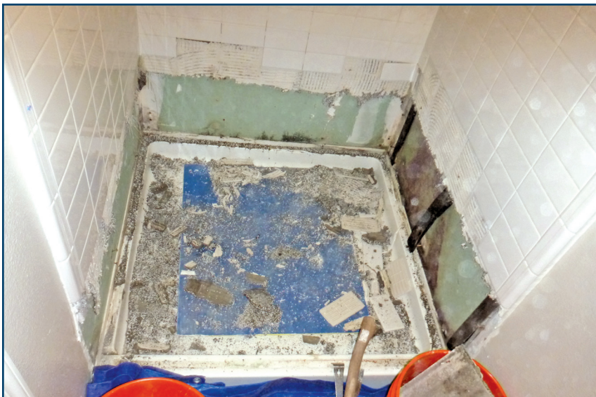
Figure 10 – Water infiltration at the CBU-to-flange transitions had damaged all walls at this purposefully selected shower.
