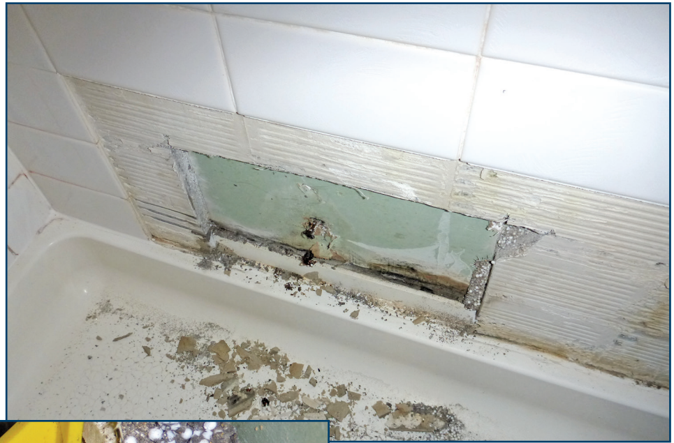
Figure 2 – Deterioration behind the loose tiles extended to the gypsum wallboard behind the CBU panels (see Figure 3).
