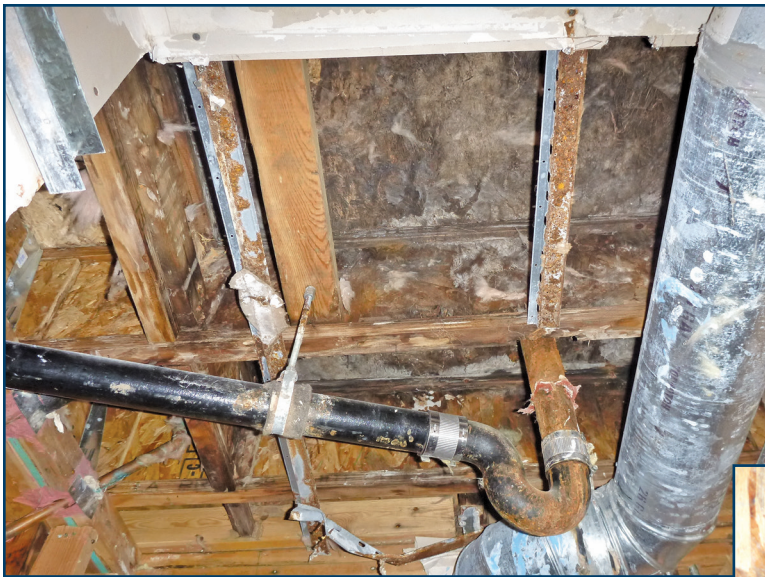
Figure 12 – Viewed (looking up) from below, structural damage resulting from the CBU butt joint leakage was severe.
