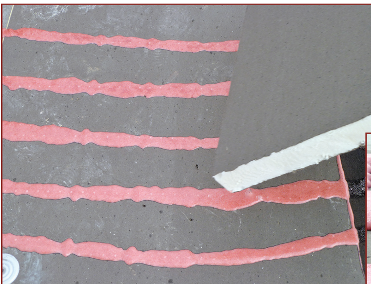
Figure 1 – Adhering a second layer of insulation over the first mechanically fastened layer.
