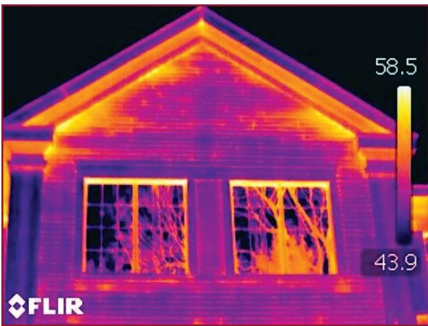
Figure 21 – Infrared image indicates air leakage.
