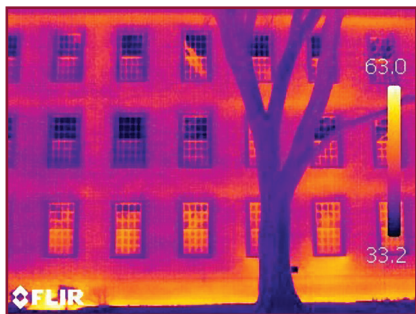
Figure 2 – Infrared image of SPF-insulated building. Note thermal bridging from uninsulated interior walls and floor slabs.
