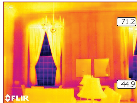
Figure 4 – Infrared image of interior space. Note thermal bridging of metal studs that bypass batt insulation.
