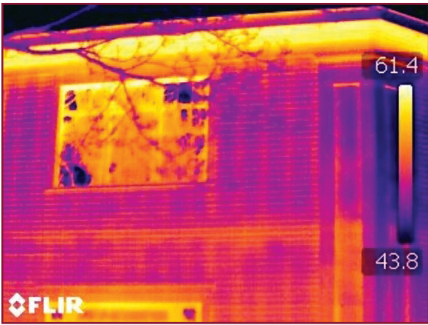
Figure 20 – Infrared image highlighting the thermal bridging caused by the metal studs.
