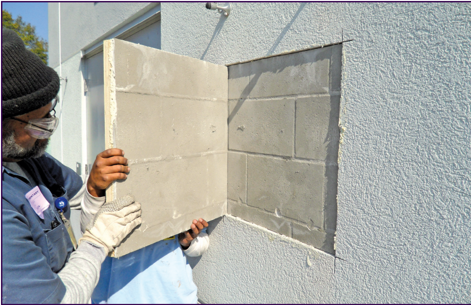
Figure 4 – Stucco test specimen after failure.
