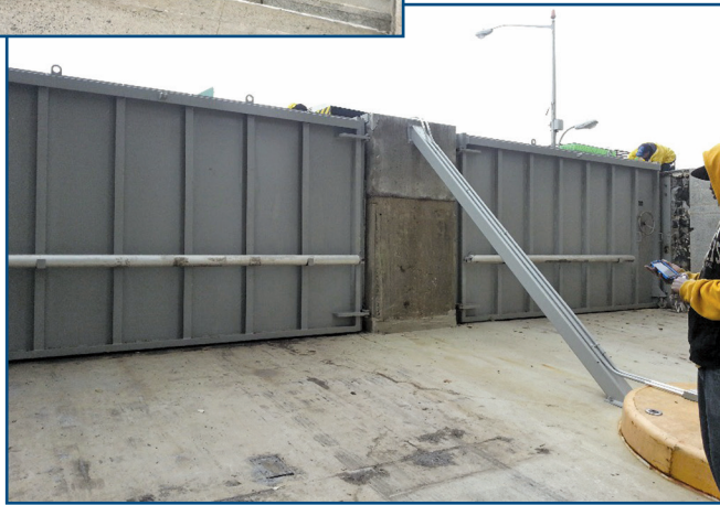
Figure 6 – Floodgates in the closed position (as seen from the “dry” side).
