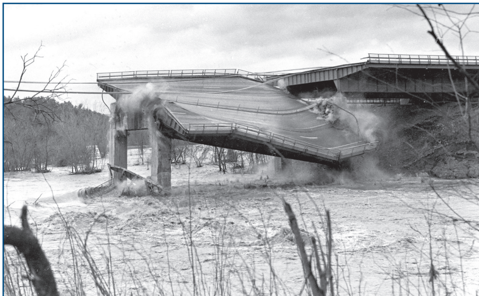
Figure 4 – Schoharie Creek Bridge collapsed suddenly in 1987 after scouring severely undermined a footing under one of the bridge's piers.
