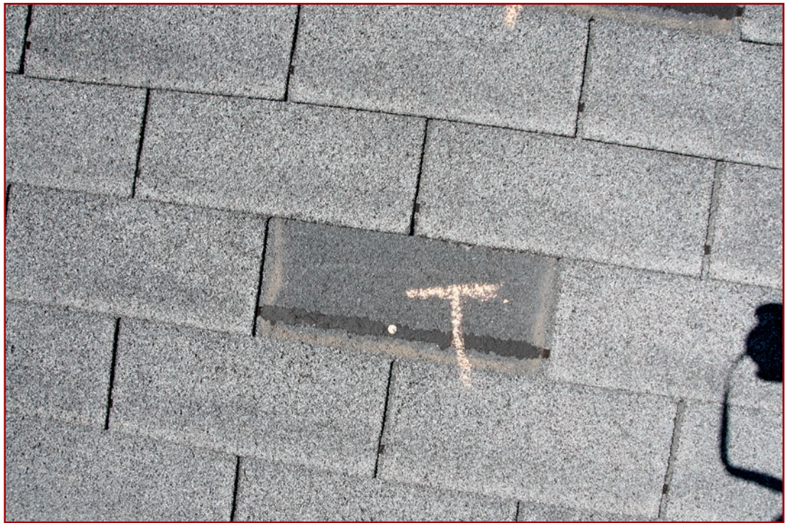
Figure 3 – Torn shingle tab.
