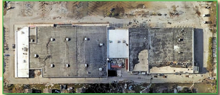
A K-Mart occupies the left end of this shopping center. Its modified-bitumen roof appears undamaged. The two mod-bit roofs at the right end (CVS and Winn Dixie) have been partially blown off.
