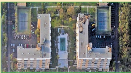
Both ends of the roof at right show visible damage to the modified-bitumen roof. The mirror image building, at left, shows no such damage. These are the "Key West at the Sea" condos on A1A, less than one mile from the end of Key West.
