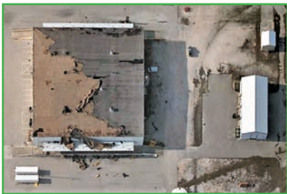
At the Key West Naval Air Station, a low-slope modified-bitumen membrane has been peeled back from half of this commercial roof. The metal canopy roofs, however, appear unscathed.
