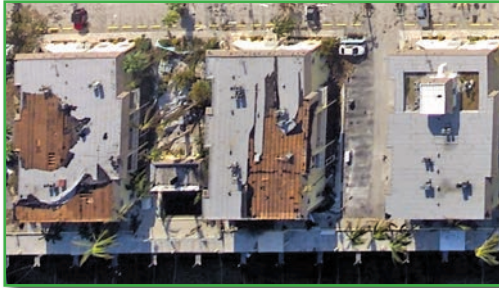
Three identical buildings and roofs: two of three mod-bit membranes show partial peel-off.
