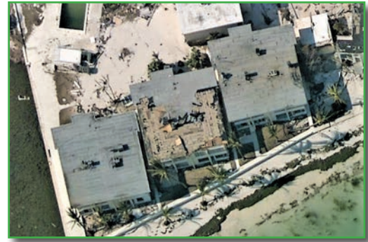
Only the center unit of these of these beachfront condos exhibited damage to its mod-bit roof.
