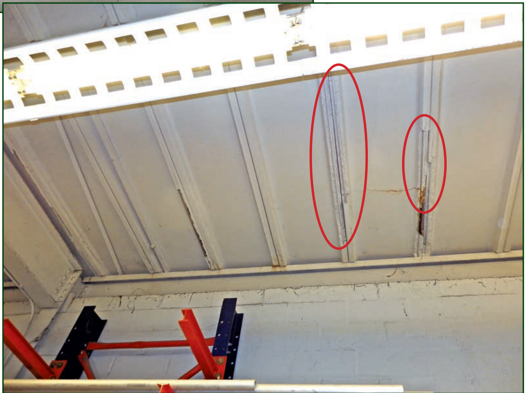
Figure 10 – Spalled concrete and exposed reinforcing steel with paint from interior renovation completed prior to storm.
