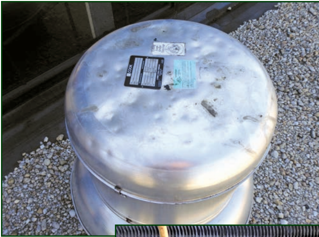
Figure 3 – Dented exhaust hood.
