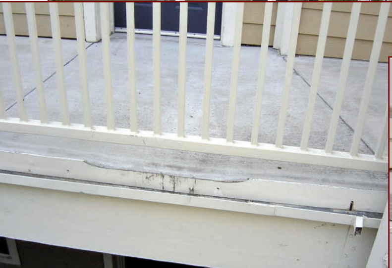
Figure 6 – Maintenance staff had carved out numerous portions of the outer edge of the T-bar flashing and concrete in order to provide drainage relief for areas of particularly problematic ponding.
