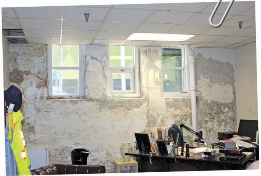
Figure 3 – Water damage on interior basement walls of east elevation, as a result of masonry, parapet wall, and roof scupper flashing defects.
