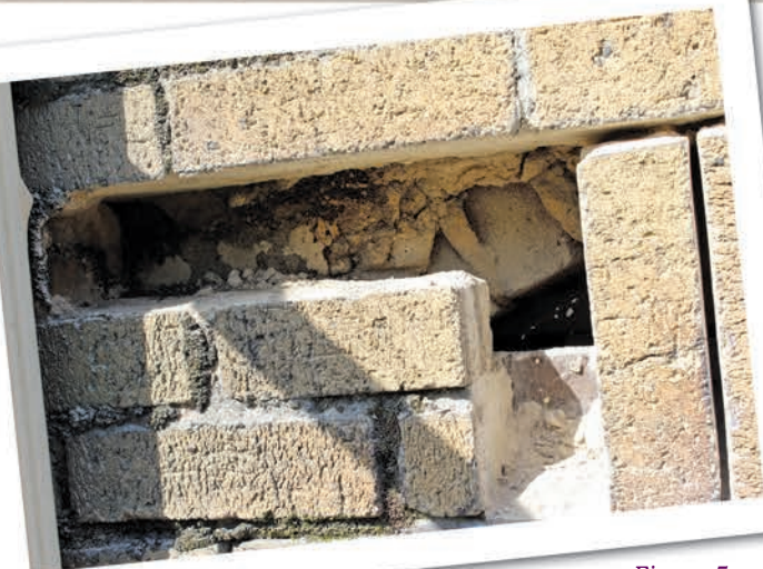
Figure 5 – Hidden arched window openings from the original façade design behind the adjoining terra cotta veneer.
