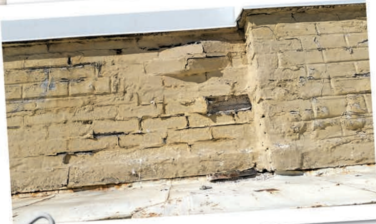
Figure 8 – Example of cracks and bulging masonry causing discontinuity of parapet wall coating.
