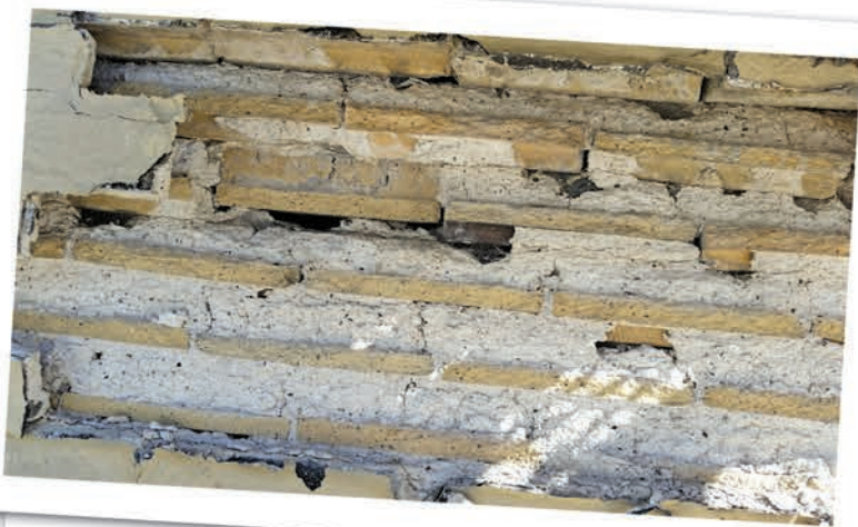
Figure 9 – Example of spalled terra cotta masonry at parapet walls.
