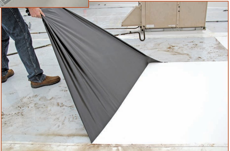
Figure 5 – Thin film covering TPO membrane. Film is removed at the completion of the installation.
