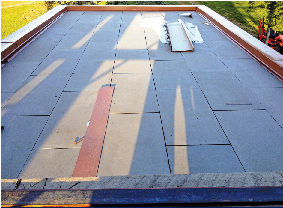
Figure 11 – A nearly finished Supra-Deck, ready for stitching screws. Bituminous roofs were commonly applied to this substrate.
