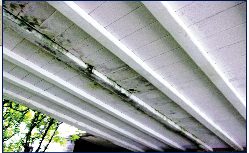
Figure 6 – This F&A System was used in a residential setting. It was a dead-flat plaza area that ponded water and leaked at cracks in the concrete topping course. Meanwhile, after decades of exposure (i.e., no topside membrane), inverted T-joists were in very good condition with no evidence of creep deflection or other distress.
