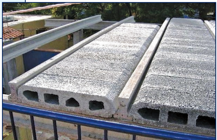
Figure 4 – Note here that the bottom face of hollow-core units is flush with the bottom of inverted T-joists. This was an alternative available to the specifier/designer.
