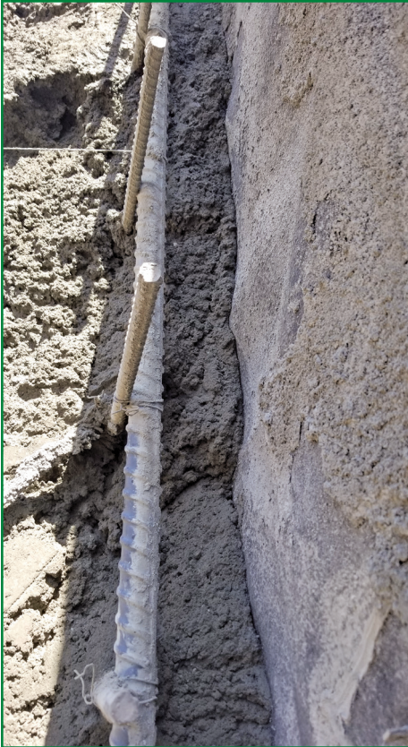
Figure 8 – View looking up and towards the edge of the shotcrete mock-up wall.
