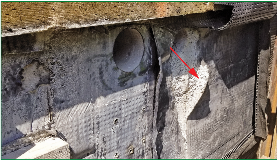
Figure 5 – Observations from the backside of the mock-up showed the membrane did not bond in the oversprayed shotcrete areas (see arrow).
