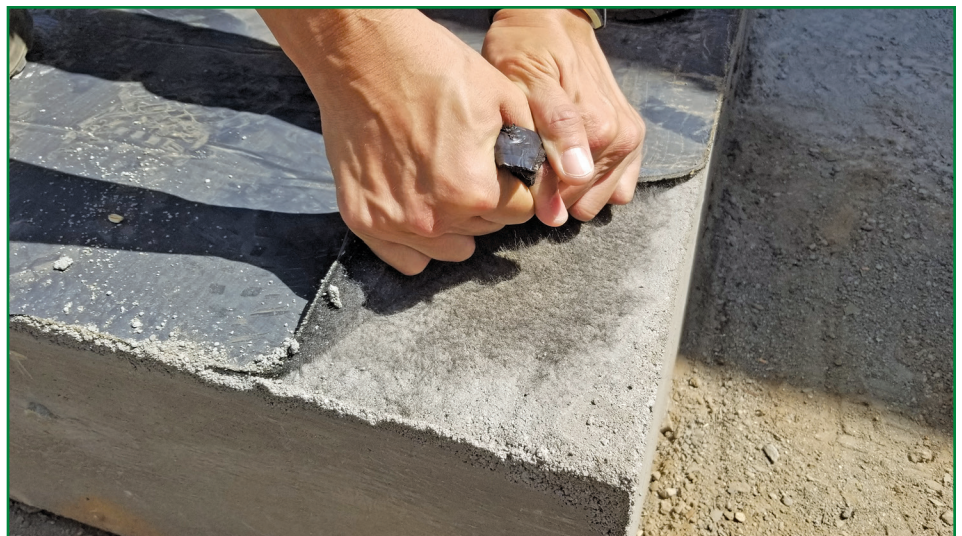
Figure 9 – Pull test of the waterproofing membrane by hand on a smaller 4- x 4-ft. mock-up.
