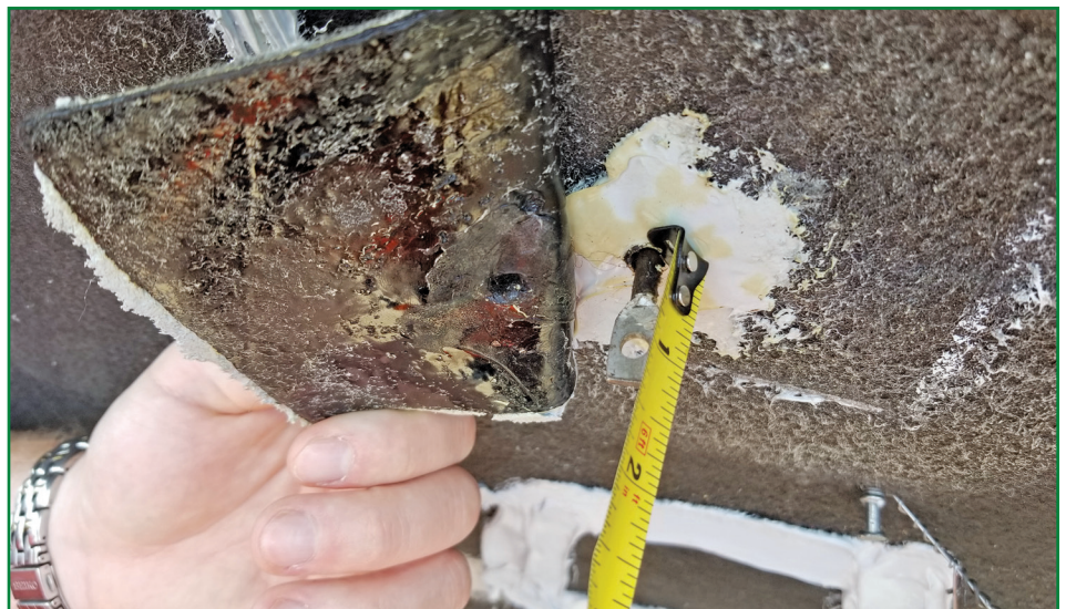
Figure 4 – Striker pin installed and detailed with waterproofing was observed to be inadequate, demonstrating a difficult detail to achieve repeatedly in the field.
