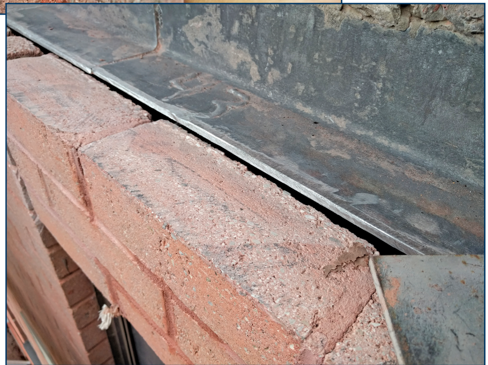
Figure 8 – No support at existing shelf angle.
