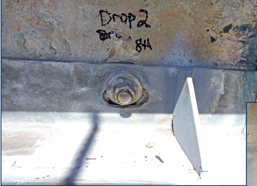
Figure 11 – Existing bolted shelf angle. Washer not making full contact due to oversized bolt slot.
