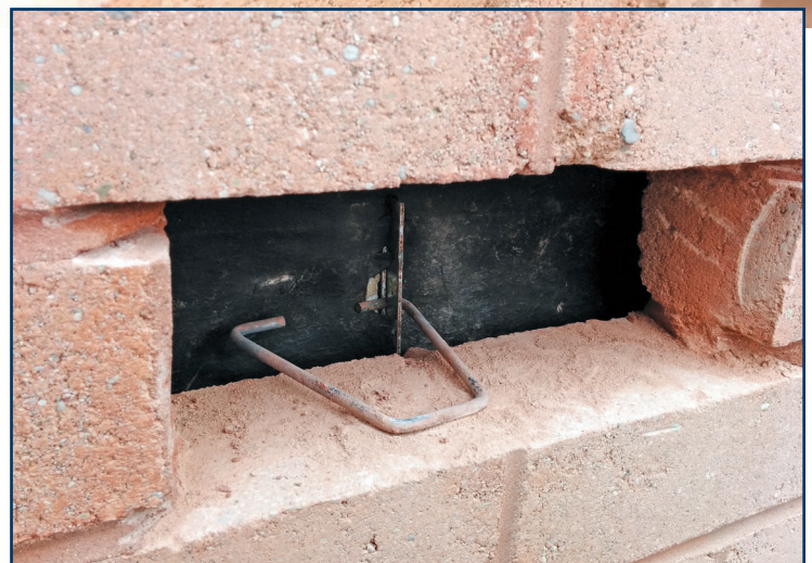
Figure 2 – Improper installation at existing wire-and-plate brick tie at steel stud backup.
