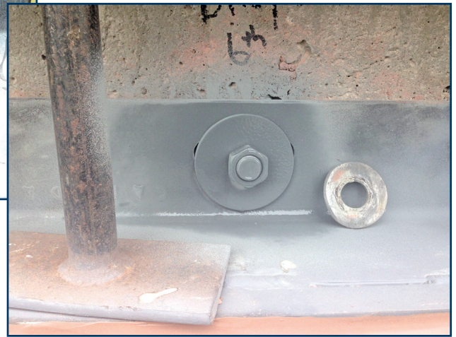
Figure 12 – Bolted shelf angle with replacement washer, making full contact with shelf angle. Original washer on right for size comparison.
