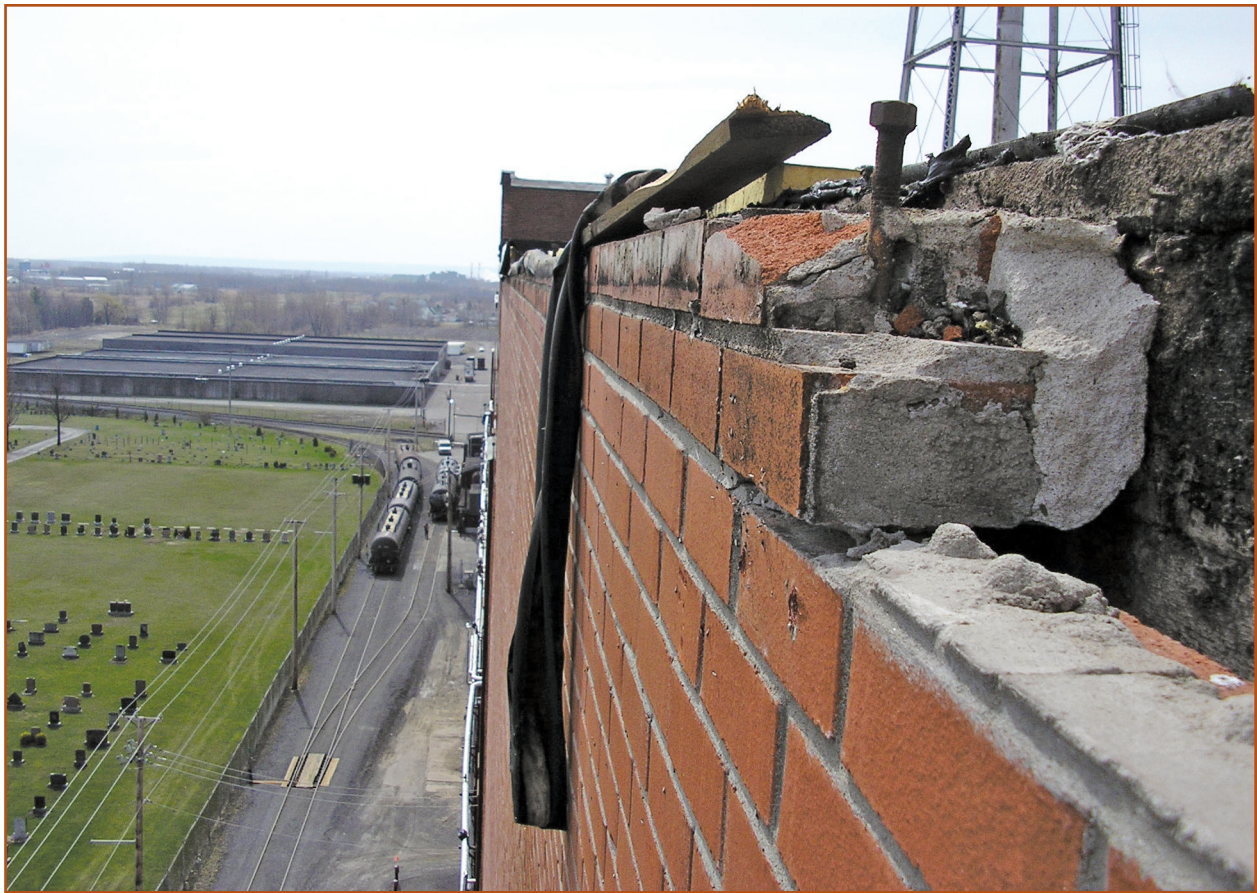
Figure 2 – Premature deterioration caused by defective connection between roof air barrier and wall air barrier. Photo courtesy of Soprema.
