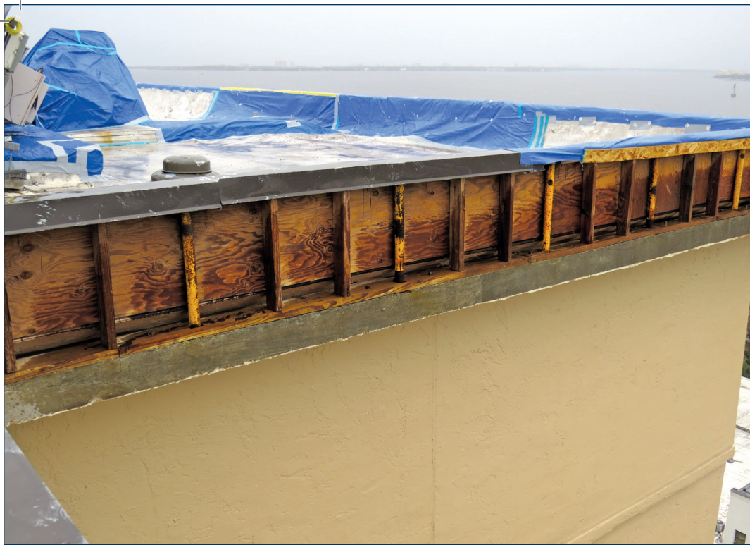
Figure 3 – Poor roof edge attachment—a major cause of failure during extreme wind events.
