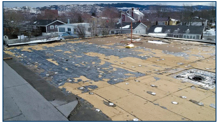
Figure 2 – Canadian East Coast roof failure during a Category 2 hurricane.
