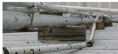
Severe damage to roof and pipe due to the use of wood blocks.
