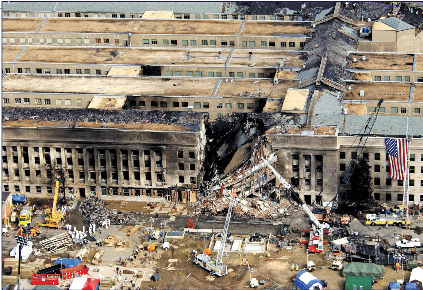
Figure 8 – Damage from impact and blast due to terrorism at Pentagon on September 11, 2001. (Image 60569, www.pixabay.com)
