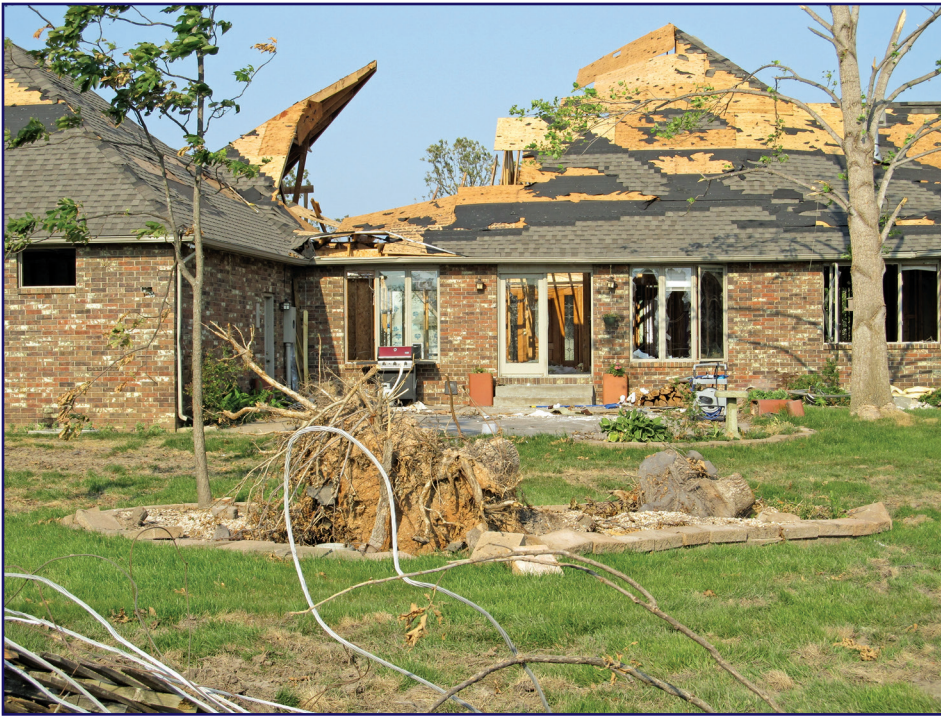
Figure 5 – Wind damage to house caused by tornado in Joplin, MO. (Image 642586, www.pixabay.com)
