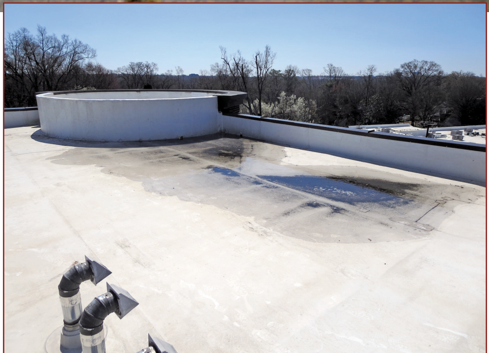
Figure 2 – Ponding typically occurs prior to reaching discharge points.
