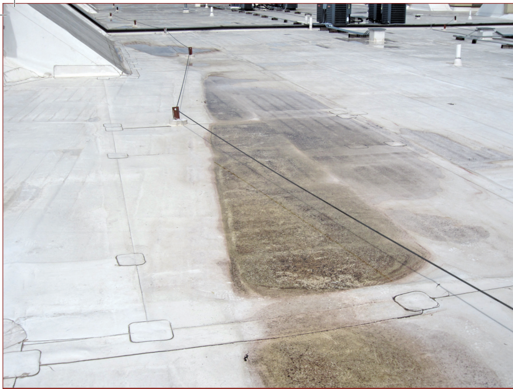
Figure 7 – Roof valley ponding.
