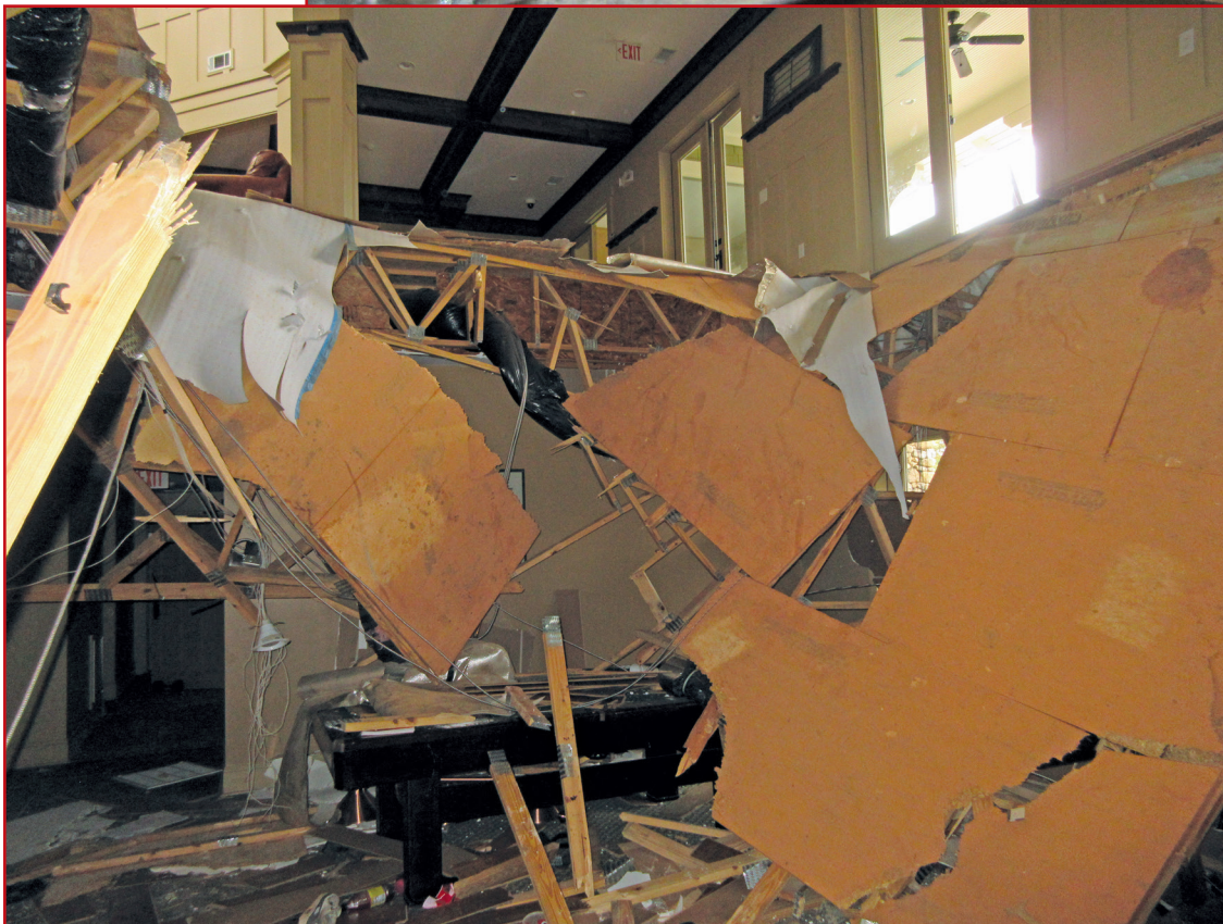
Figure 3 – View of collapsed floor framing.
