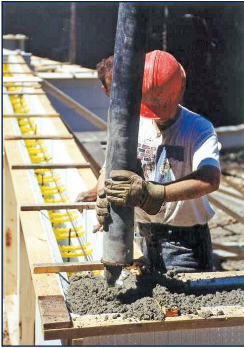
Figure 5 – Concrete is typically placed in ICF walls using a boom pump. Photo courtesy of Quad-Lock.
