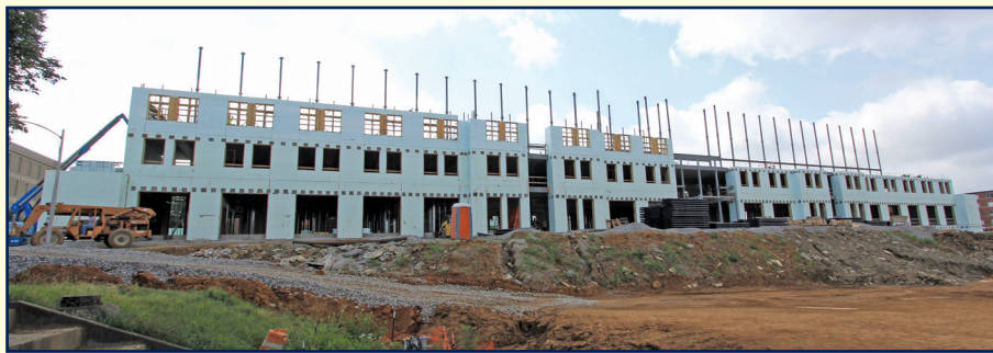
Figure 18 – Martin Hall at Eastern Kentucky University under construction. Image courtesy of Nudura.
