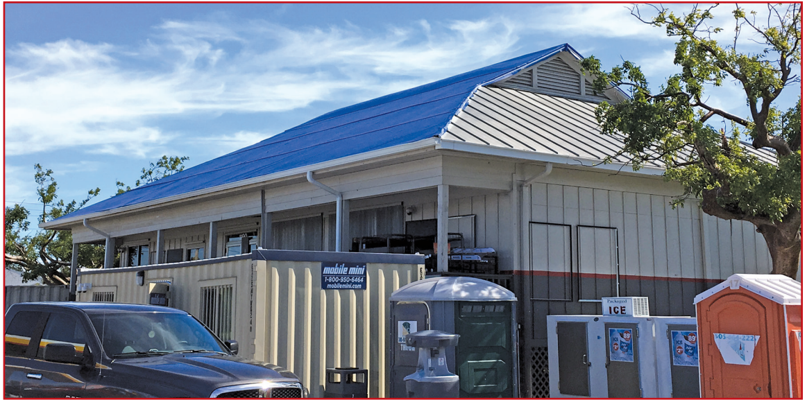
Figure 4 – Damaged architectural standing-seam roof on convenience store.
