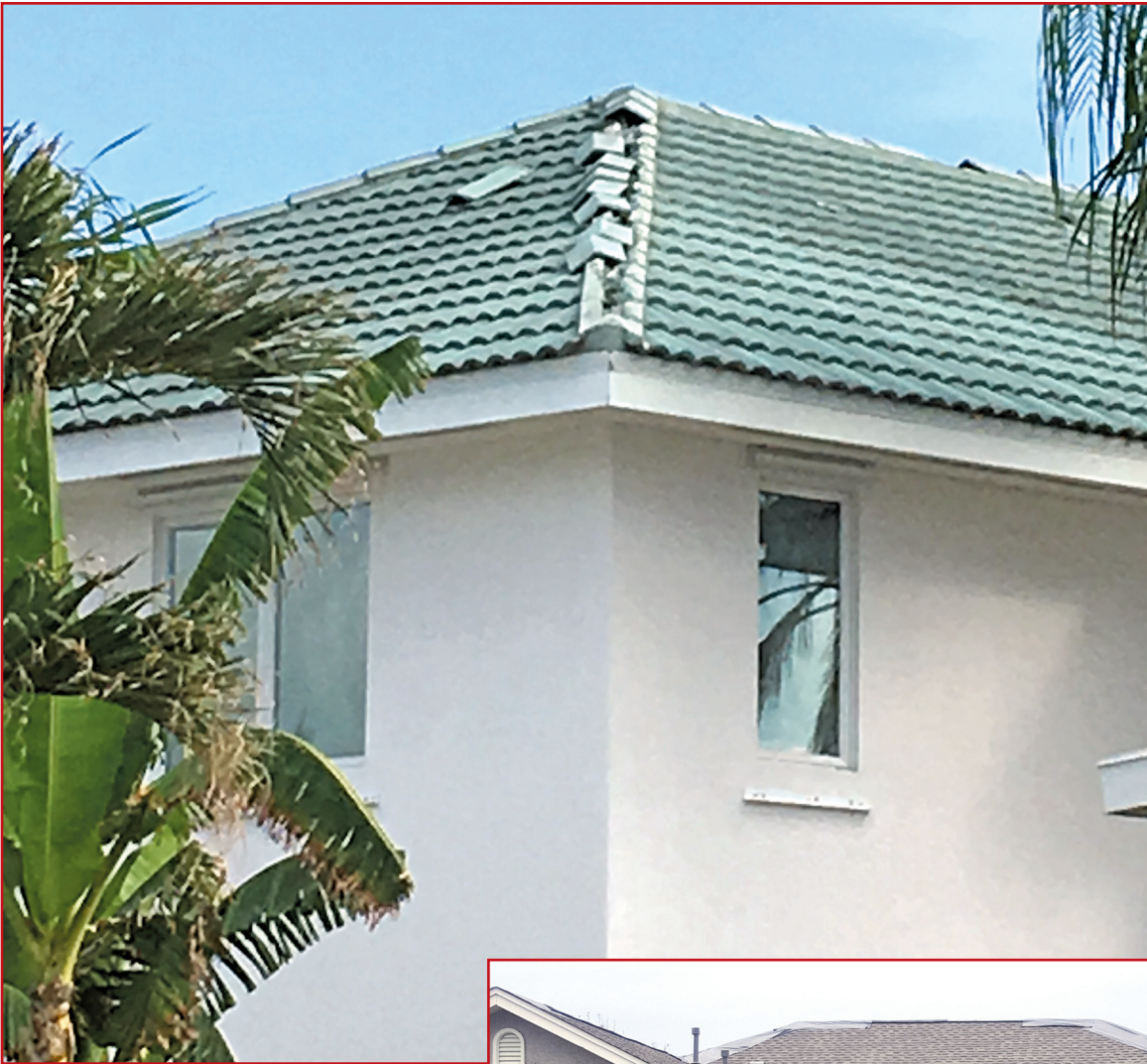
Figure 2 – Hip damage to tile roof. Courtesy of ARMA.
