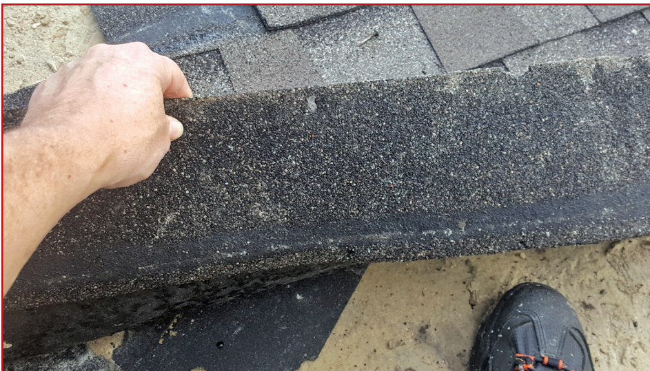
Figure 5 – Damaged asphalt shingle showing incorrect fastener location. Courtesy of ARMA.
