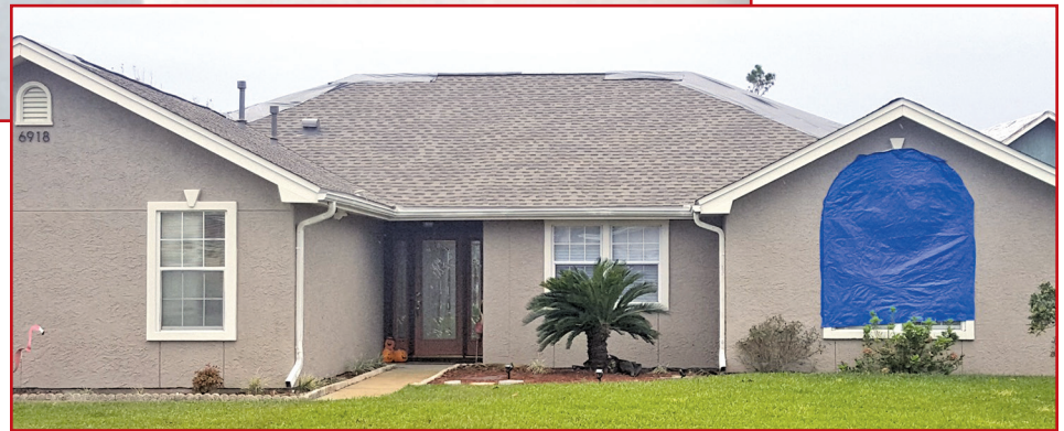
Figure 3 – Hip and ridge damage to asphalt shingle roof. Courtesy of ARMA.
