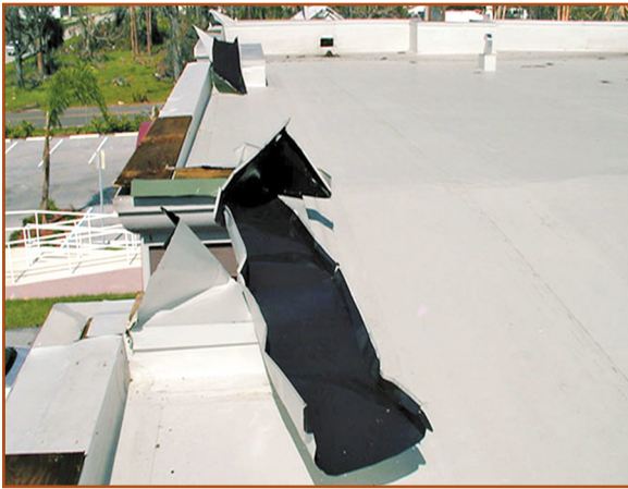
Figure 2 – Studies of roofing damage conducted by RICOWI, in conjunction with FM and SPRI, reported that nearly 60 percent of damaged roofs were caused by failure at the perimeter.
