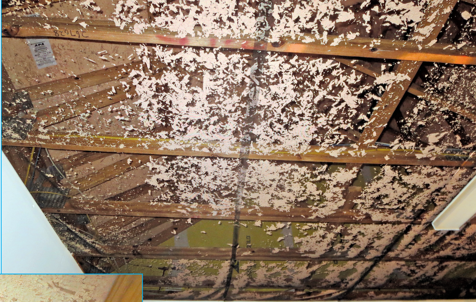
Figure 6 – Screen placed to catch fire-resistant paint shown falling from the OSB roof deck in Figure 5.
