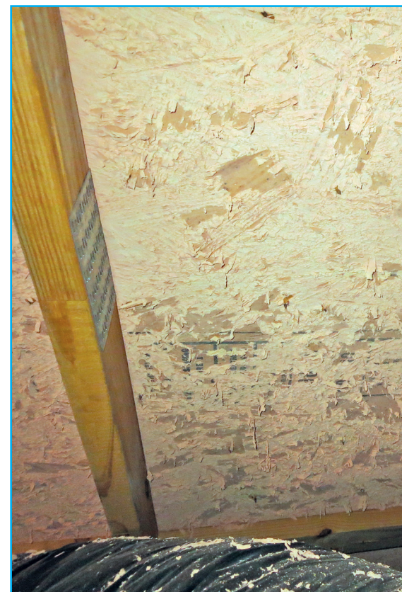
Figure 5 – Adhesion failure of fire-resistant paint.
