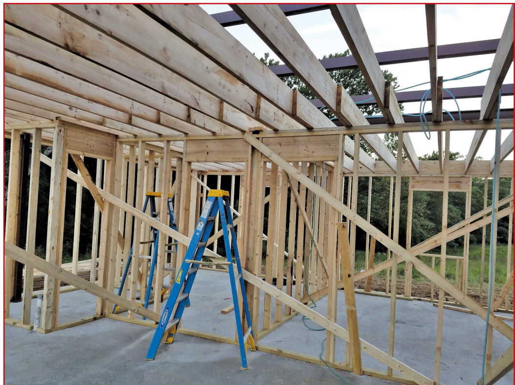
Figure 3 – Everyone needs to be lifting in the same direction for a wall to be properly constructed.
