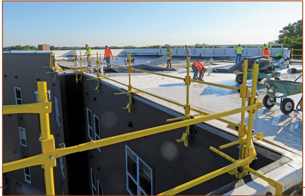
Figure 15 – Perimeter safety rails.
