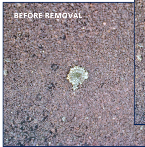
Figures 2 and 3 – These photos were contributed by Tim Wrigley of IKO Industries. He lifted the lichen shown in the immediate right, and the granules and top layer of asphalt came away with the lichen, leaving the pothole shown in the far right.
