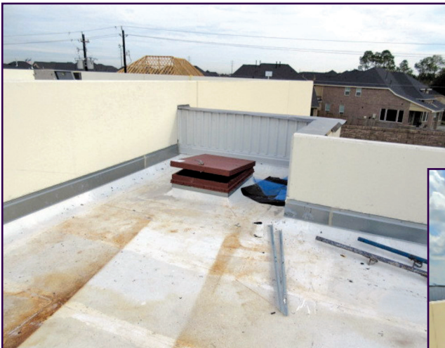
Figure 4 – Corrosion stains from sheet metal storage on cap sheet.
