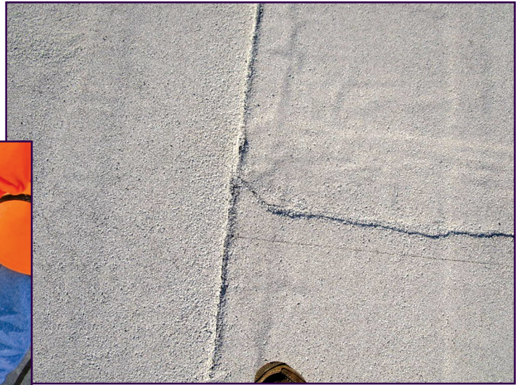
Figure 8 – Rounded corner of cap sheet and granules embedded in bleed-out.
