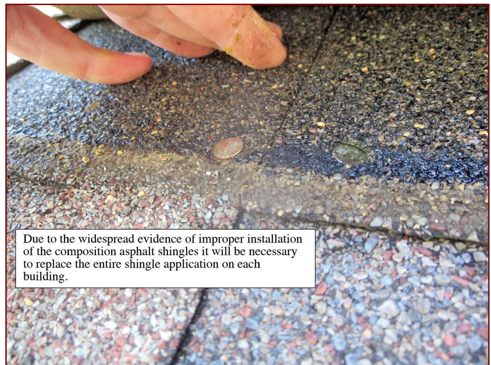
Figure 6 – Example of “widespread” improper shingle installation used to support the recommendation of complete roof replacement.
