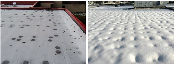
Figure 1 – Visual impact of thermal bridging of roofing fasteners (courtesy: RCABC).
