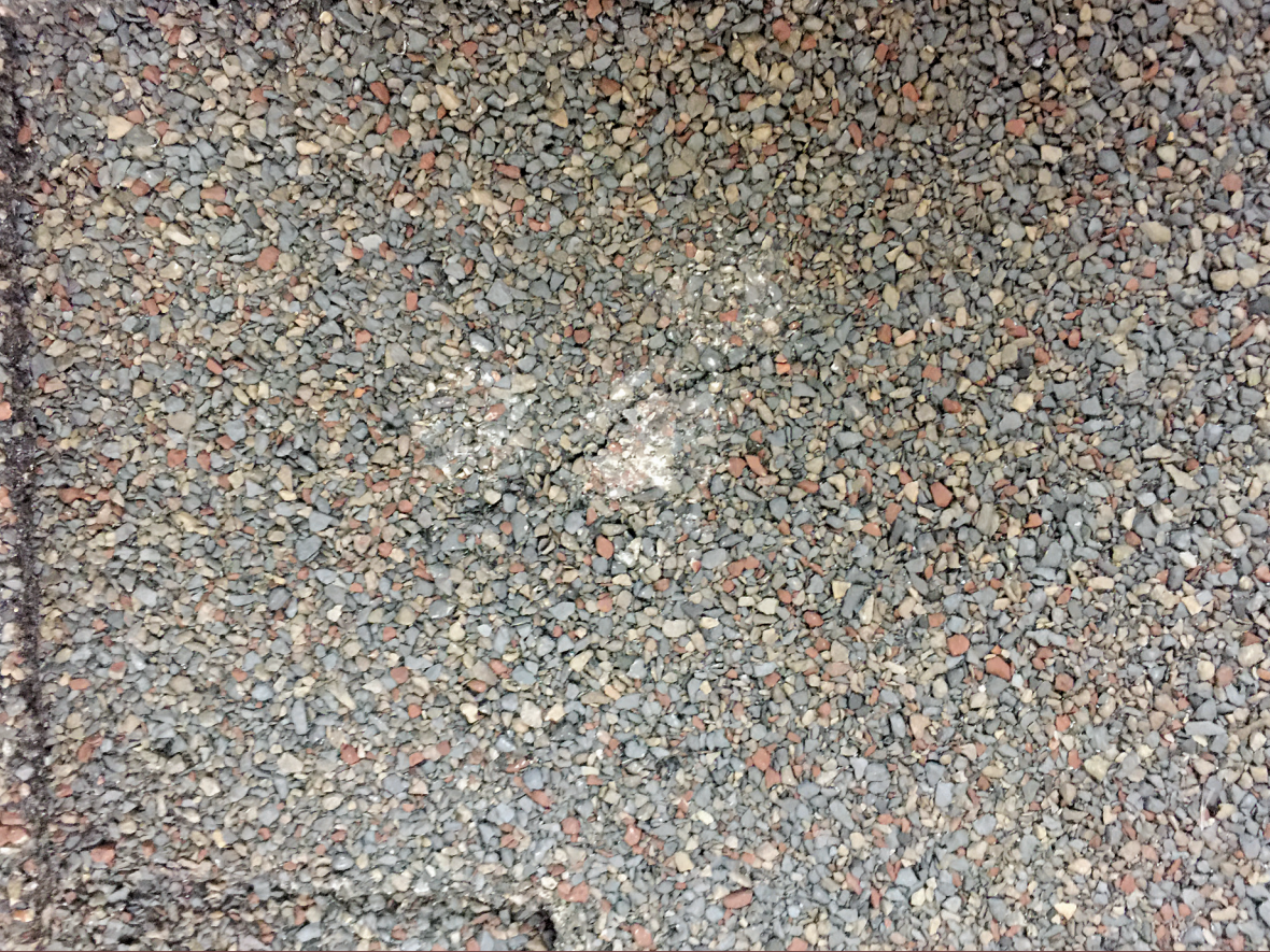
Figure 8 – Crack in the shingle after performing UL 2218 steel ball drop test.
