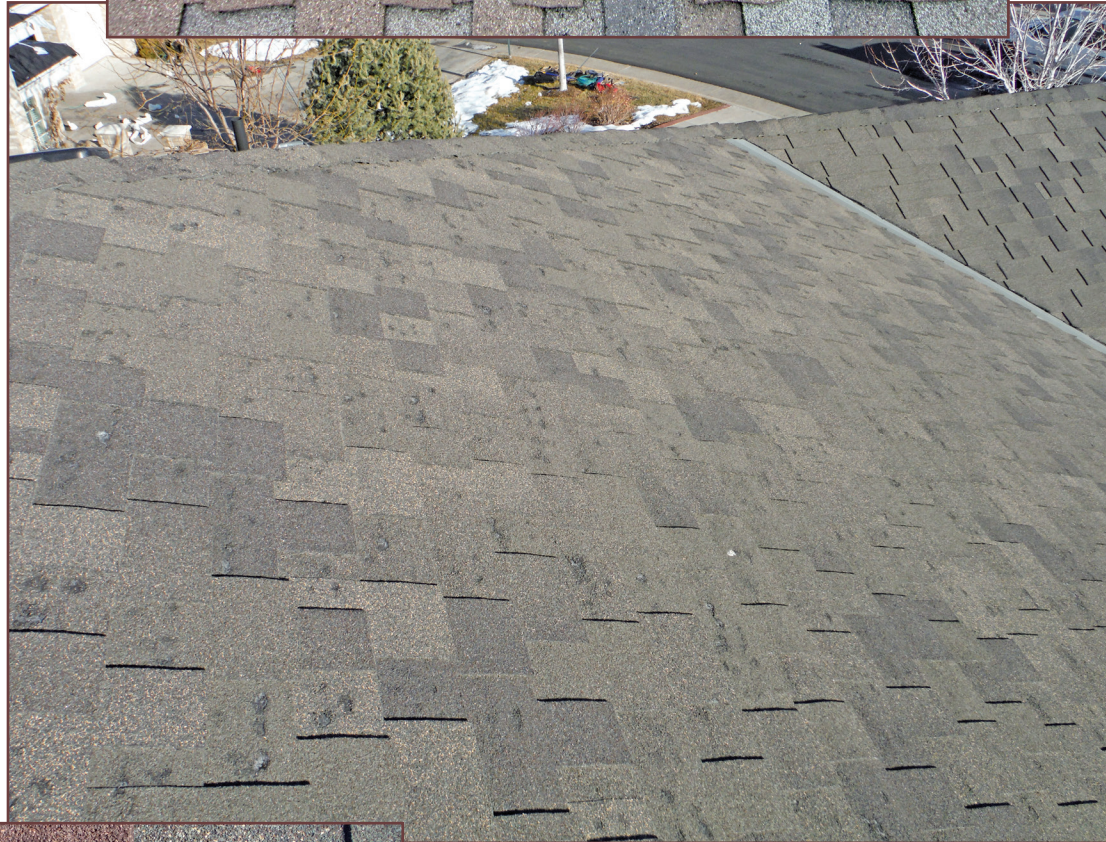
Figure 3 – Visible, patterned hail damage at the notches of shake-style shingles.
