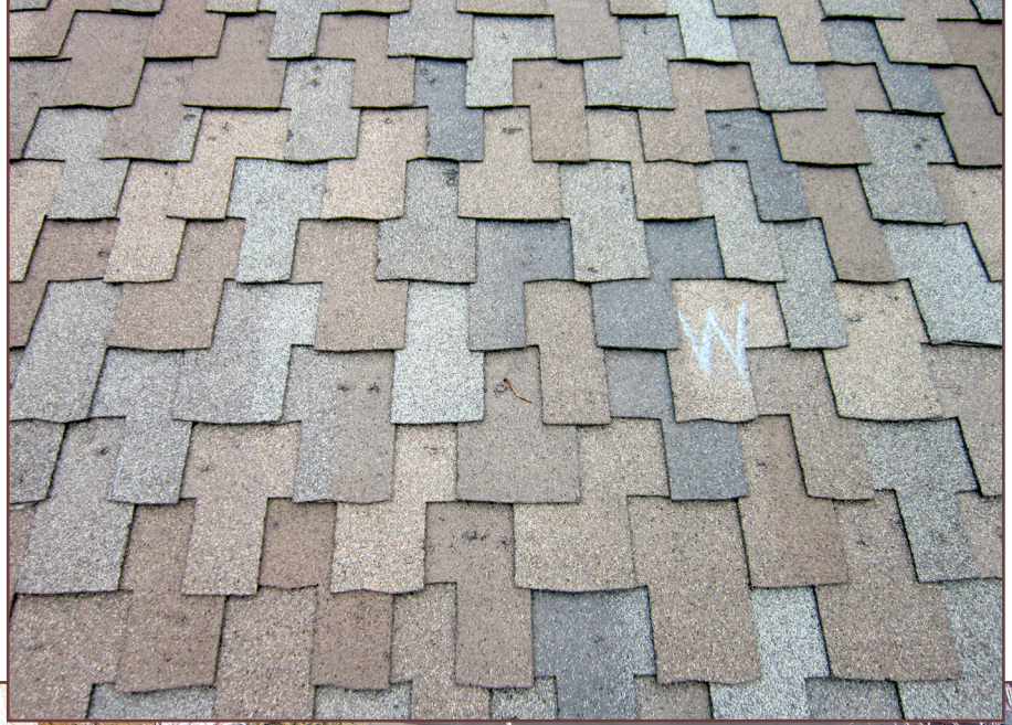
Figure 2 – Visible, patterned hail damage at the notches of shake-style shingles.
