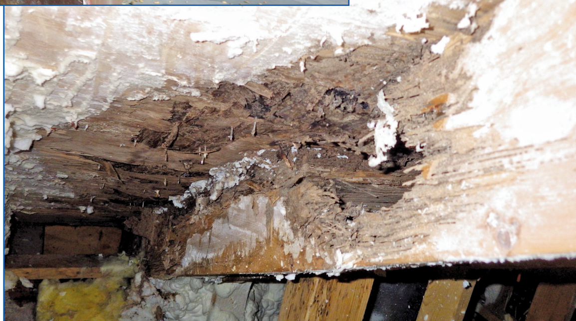
Figure 6 – Water-damaged roof deck at chimney.
