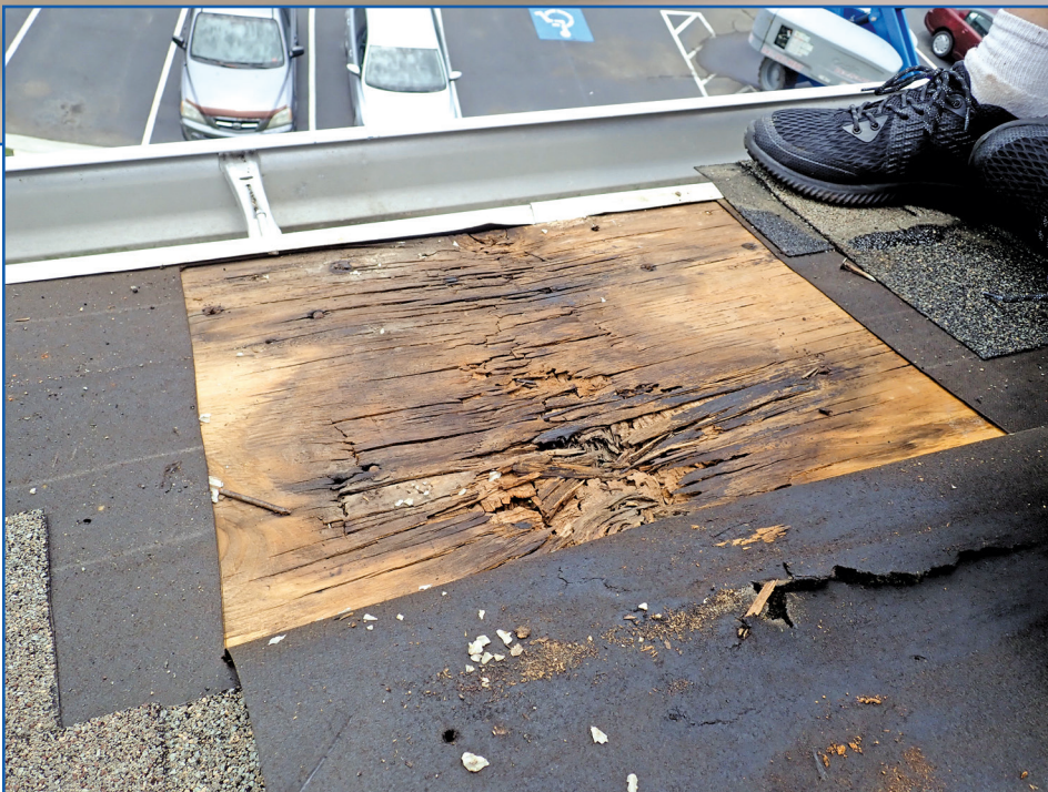
Figure 14 – Water damage at roof eave.
