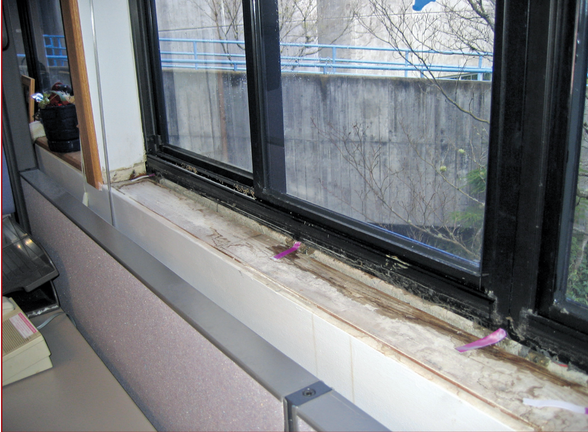
Figure 1 – Water leakage paths indicated by pink paper strips at interior after removal of wood stool.
