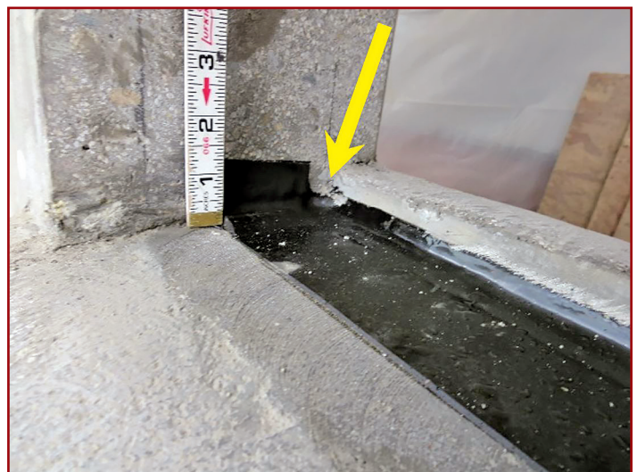
Figure 22 – Voids found in waterproofing mock-up at inside corners (arrow).
