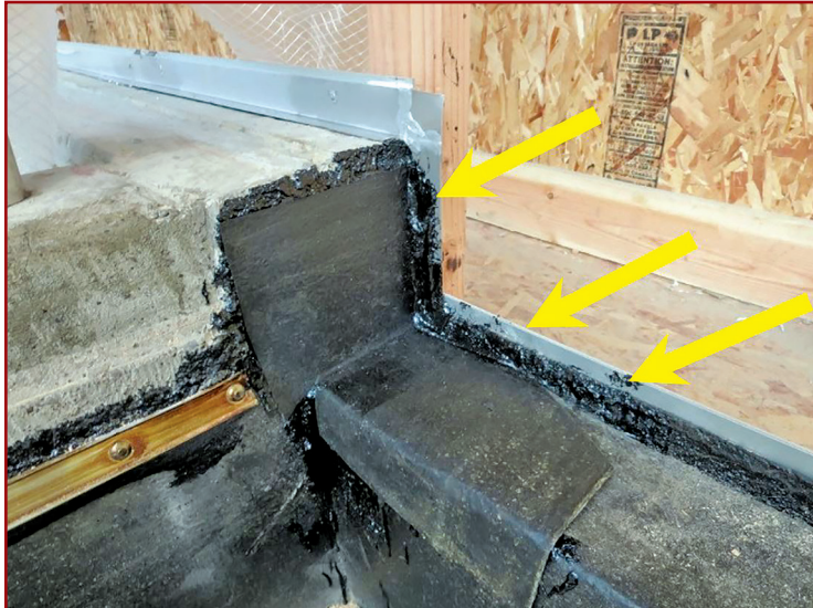
Figure 20 – Fully bonded waterproofing membrane application at window curb. Arrows indicate metal bracket back dam. Note: protection layer is present on top of waterproofing membrane.
