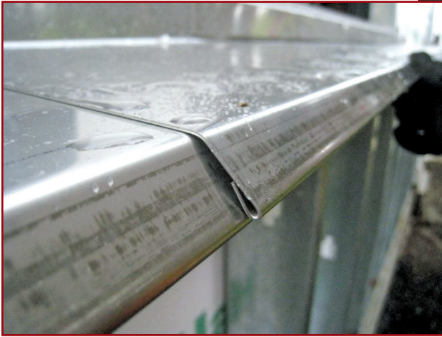
Figure 7 – Hemmed drip edge not properly integrated with adjacent flashing component at lap.
