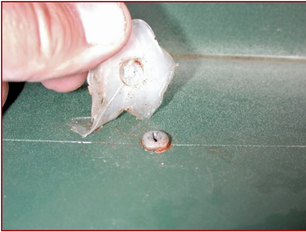
Figure 11 – Sealant debonded from fastener head at metal pan.
