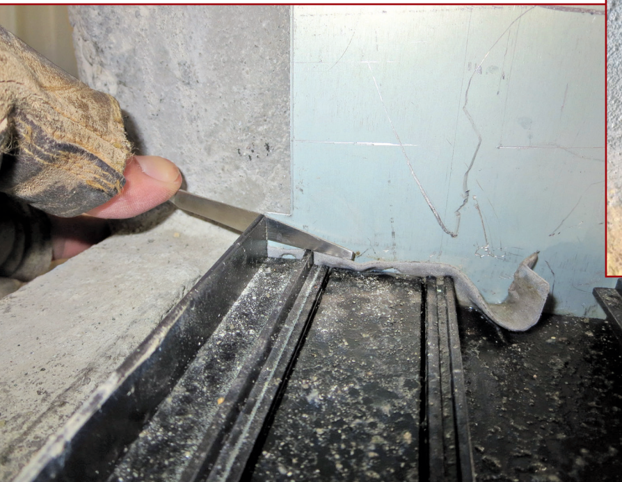
Figure 13 – Damaged foam gasket and gap between back dam and end dam.
