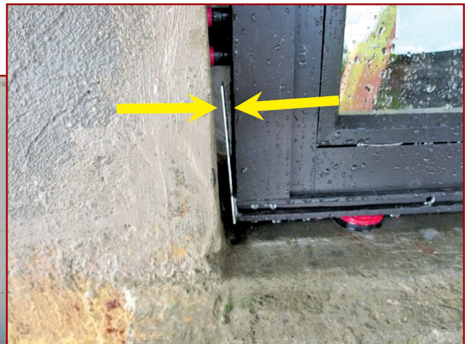
Figure 14 – Gap between top of end dam and window jamb.
