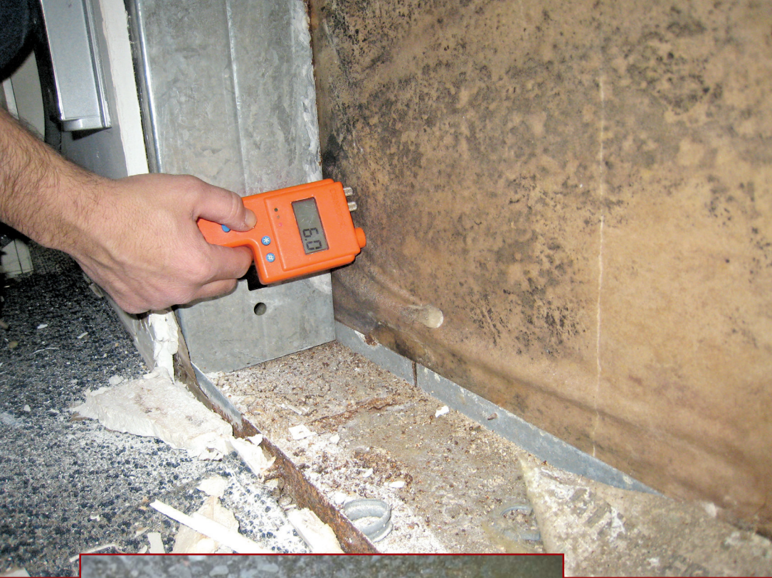
Figure 3 – Cavity side of exterior gypsum sheathing displays organic growth and rippling (debonding) of the paper facing.
