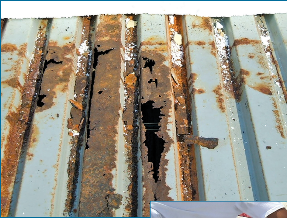
Figure 5 – Damaged section of roof deck.
