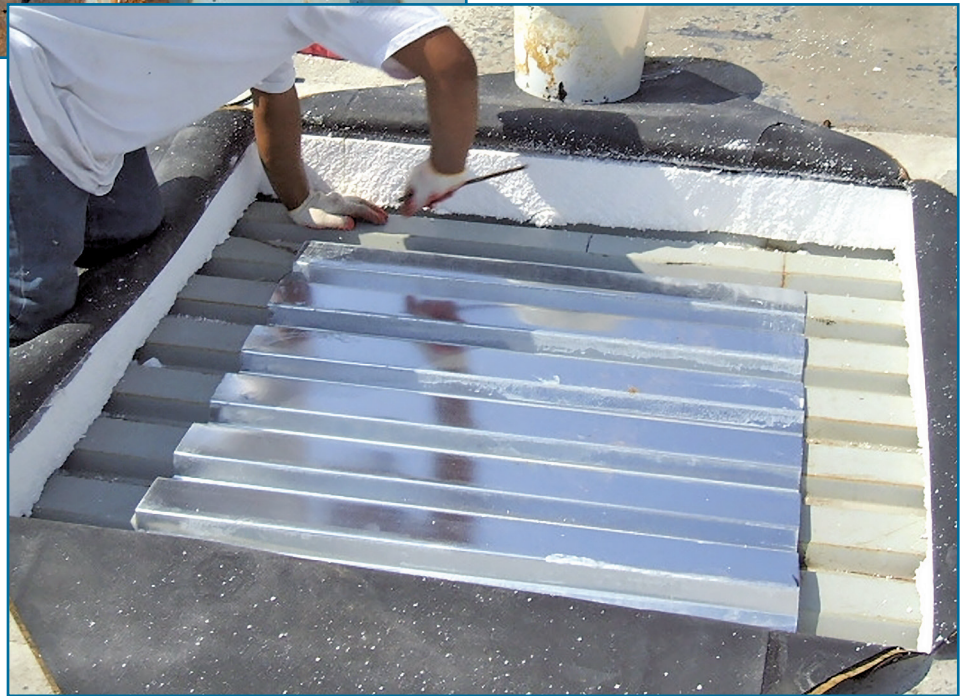
Figure 6 – Repaired section of damaged roof deck (performed prior to contractor’s use of any roofing products on the project).
