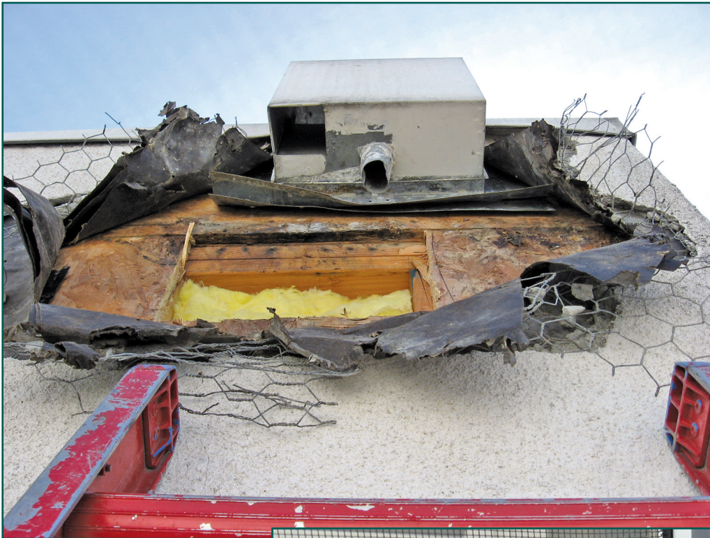
Figure 1 – In 2007, six experts from separate building envelope consulting firms climbed this ladder on behalf of six separate law firms and five separate insurance carriers to document conditions exposed by defense testing.
