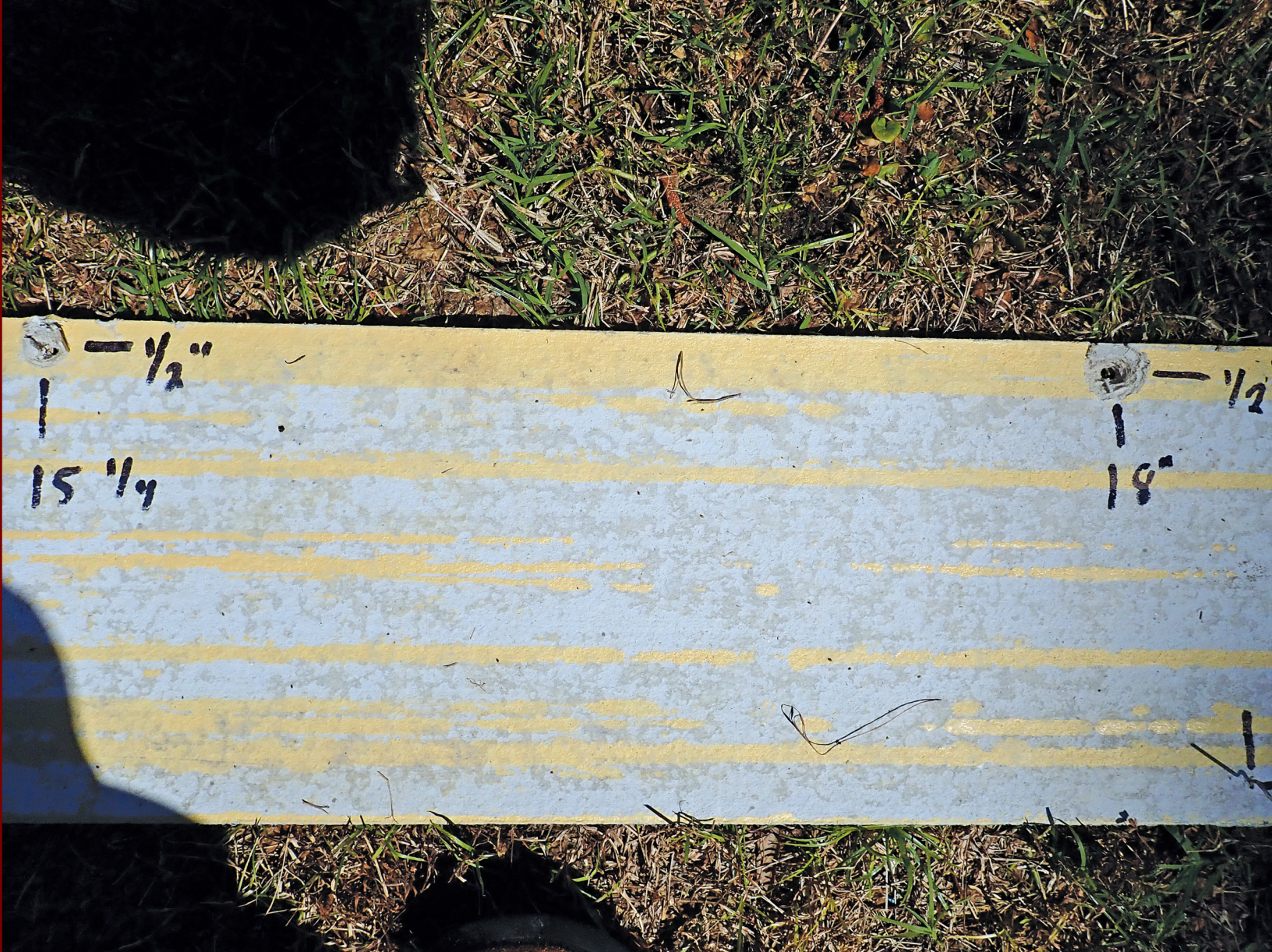
Figure 5 – View of improper horizontal on-center fastener spacing.
