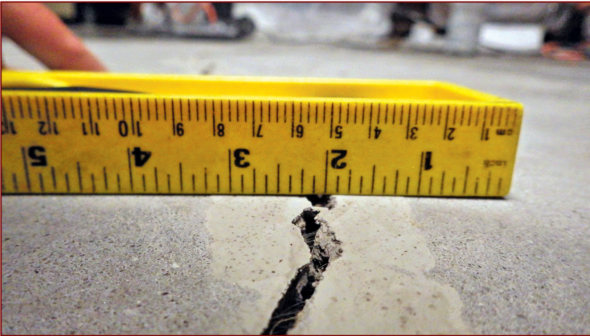
Figure 6 – View of cracking in a reinforced concrete slab-on-grade foundation.
