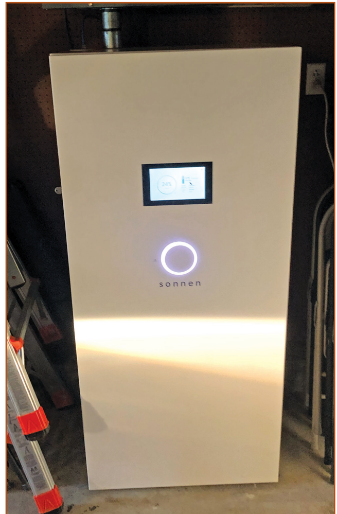
Figure 2 – Typical ESS installed in residential garage. Image courtesy of GBH International.
