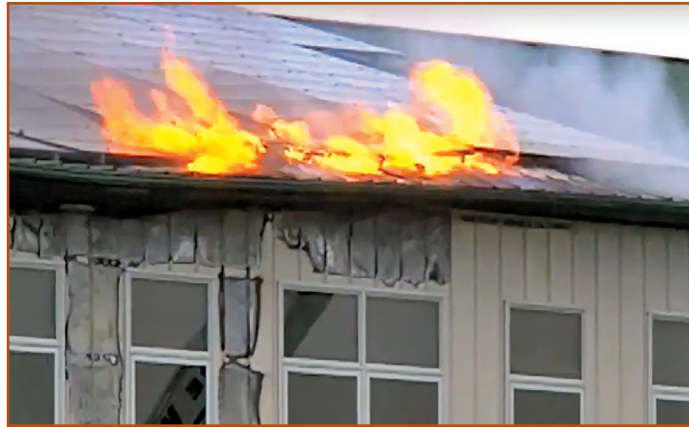
Figure 6 – PV panels burning on roof of Organic Valley Dairy headquarters, by WXOW News.
