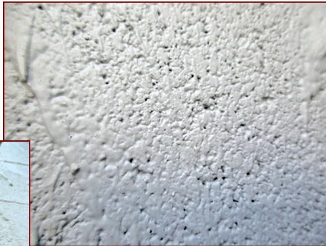
Figure 12 – Voids in fluid-applied air barrier on porous CMU.
