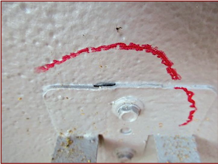
Figure 15 – Void in fluid-applied air barrier at top edge of masonry anchor plate.
