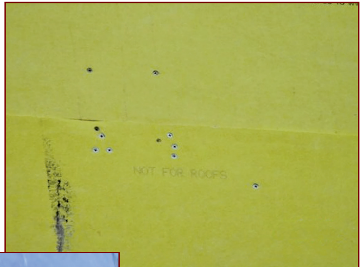
Figure 10 – Improperly positioned fasteners in sheathing.
