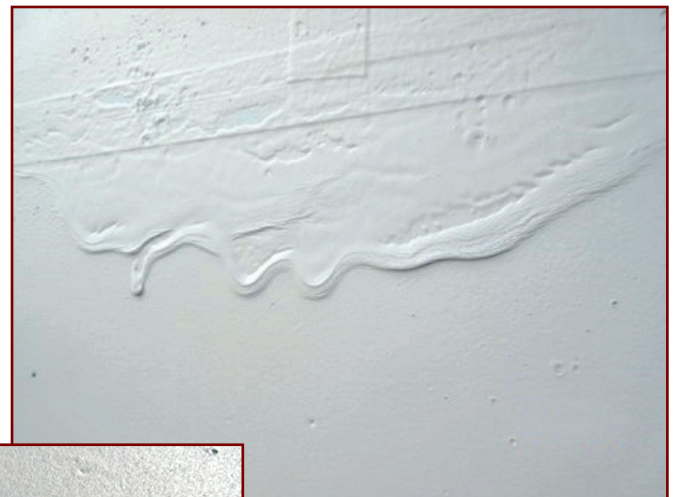
Figure 4 – Sloughing of excessive application of fluid-applied air barrier.
