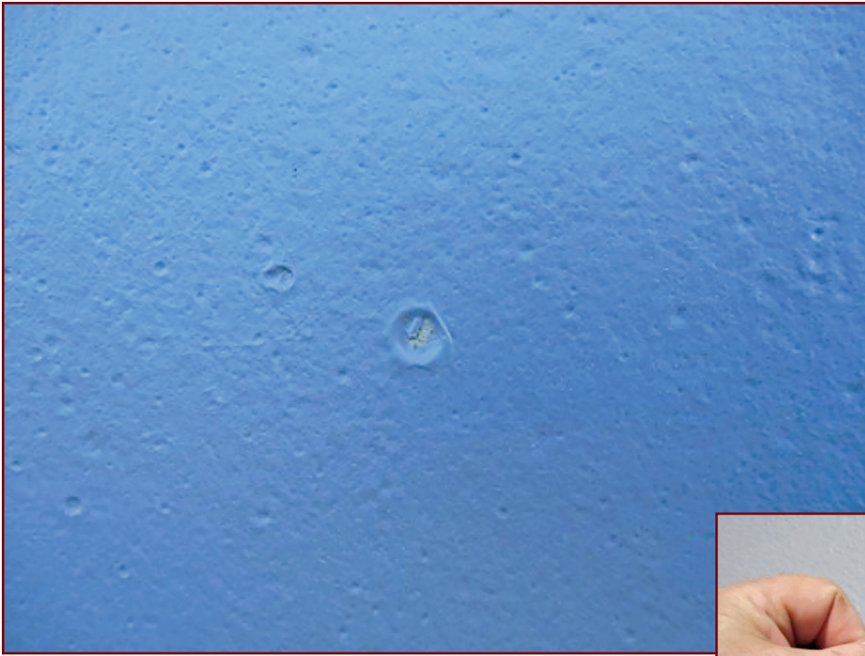
Figure 6 – Close-up view of a crater in surface of fluid-applied air barrier.
