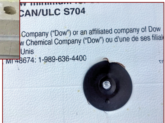
Figure 18 – Damaged foil facer on insulation used as WRB around over-driven fastener.
