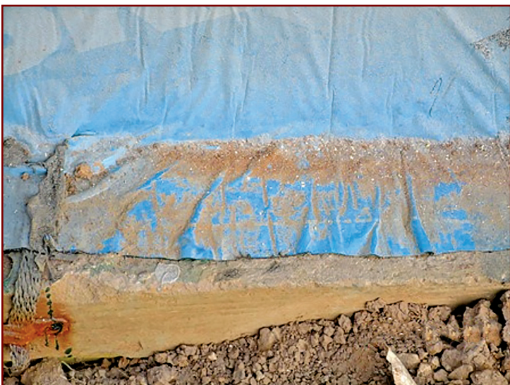
Figure 8 – Soil-contaminated base of wall.
