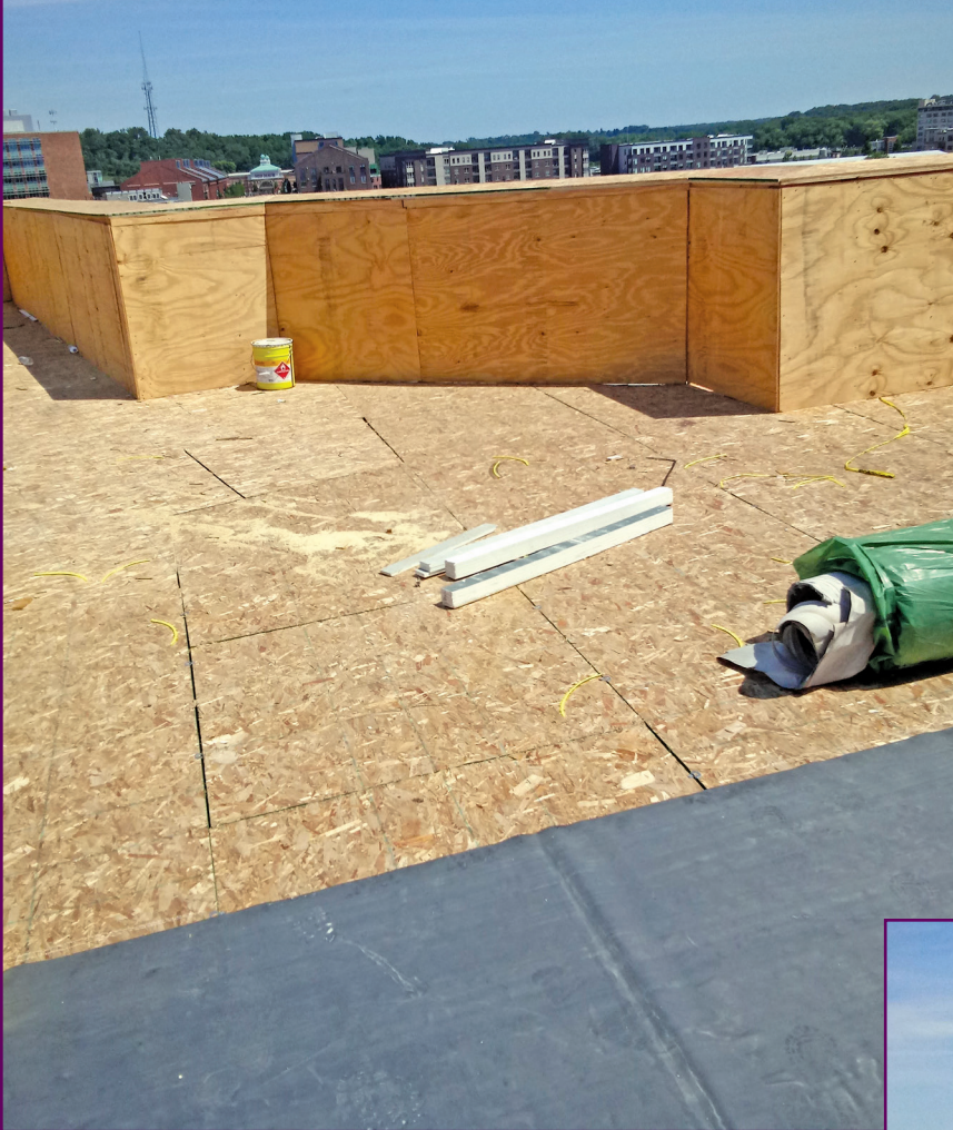
Figure 3 – Case Study 2 – No insulation over OSB decking.
