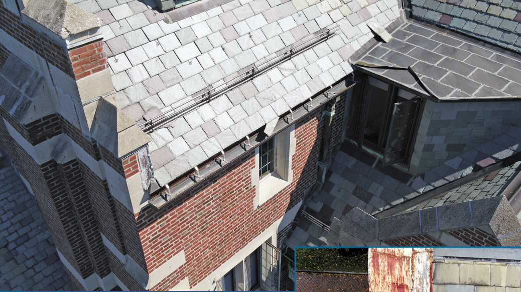
Figure 8 – UAV images of sloped, gable-style roofs covered with slate. The roof has lead-coated copper valley and ridge flashings. The one on the left has hung copper gutters and a snow rail system.
