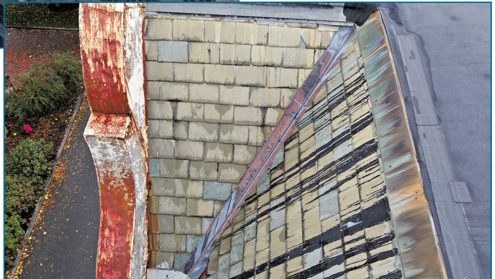
Figure 9 – This roof was previously surveyed in 2019. A large New England campus was imaged using unobtrusive UAVs. Shown is the sloped gable-style roof covered with slates that had undergone considerable damage.
