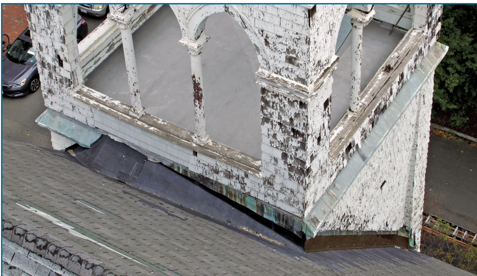
Figure 10 – Church with significant damage imaged using a UAV in lieu of a bucket truck due to safety issues. Amongst many issues, damage was observed in an inappropriately sized cricket. The cricket should divert water from the high roof around the chimney.
