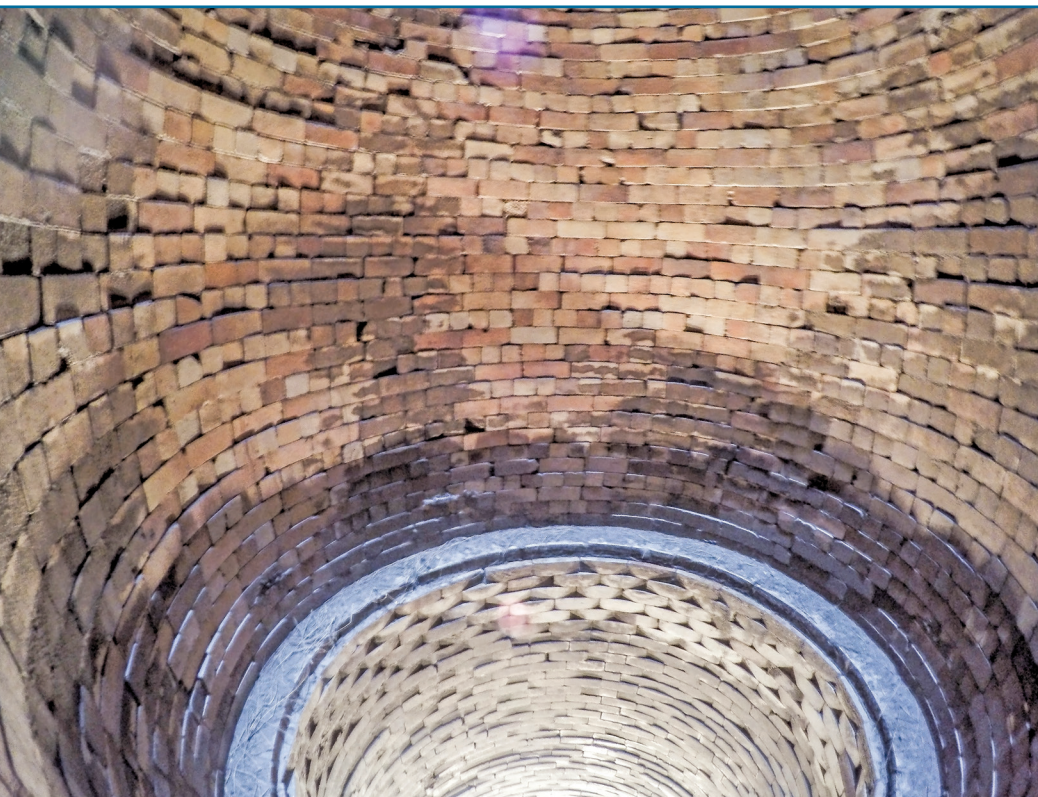
Figure 5 – Interior of an uncapped industrial smokestack as imaged by a custom-built UAV.
